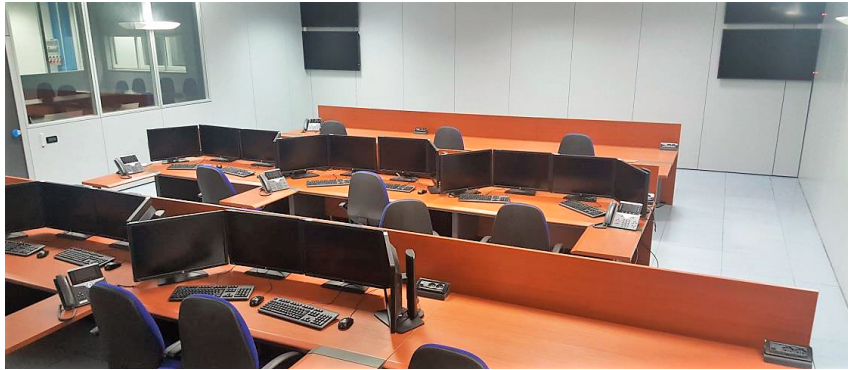
Figure 4.11: ROCC Main Operations Control Room (Credit: ALTEC).
