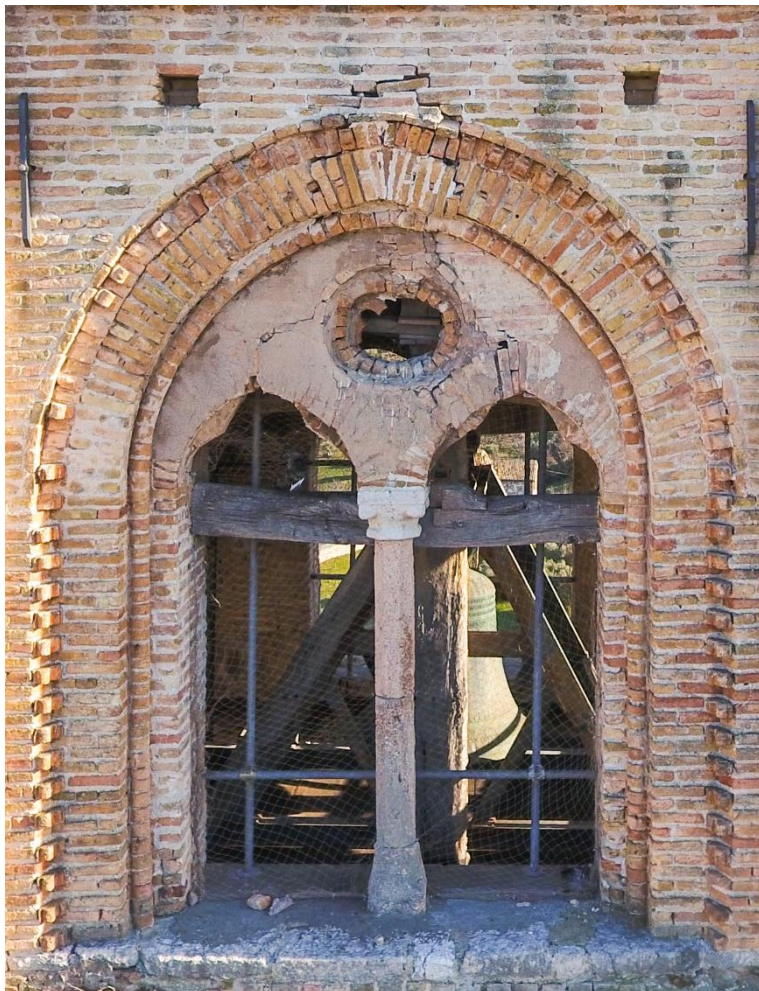
Image of the west facing double lancet window of the Duomo Vecchio di San Severino, damaged by the earthquake swarm of august 2016.
