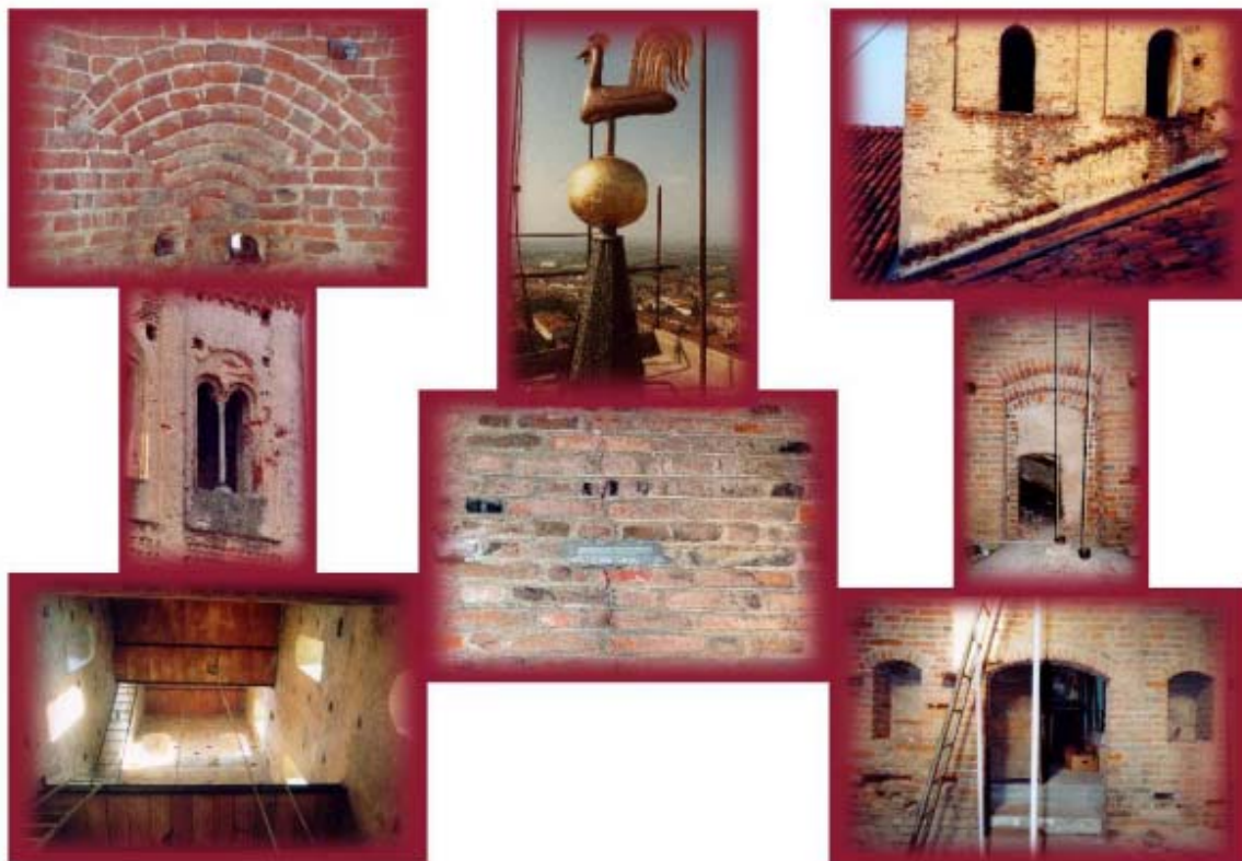
The state of the bell tower during the preparation of the thesis
