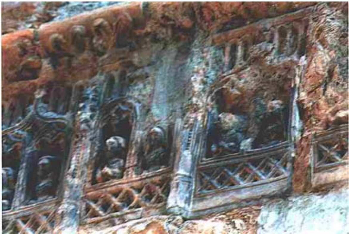
Conte Verde's house, Rivoli (Turin). Particular of the brick's deterioration
