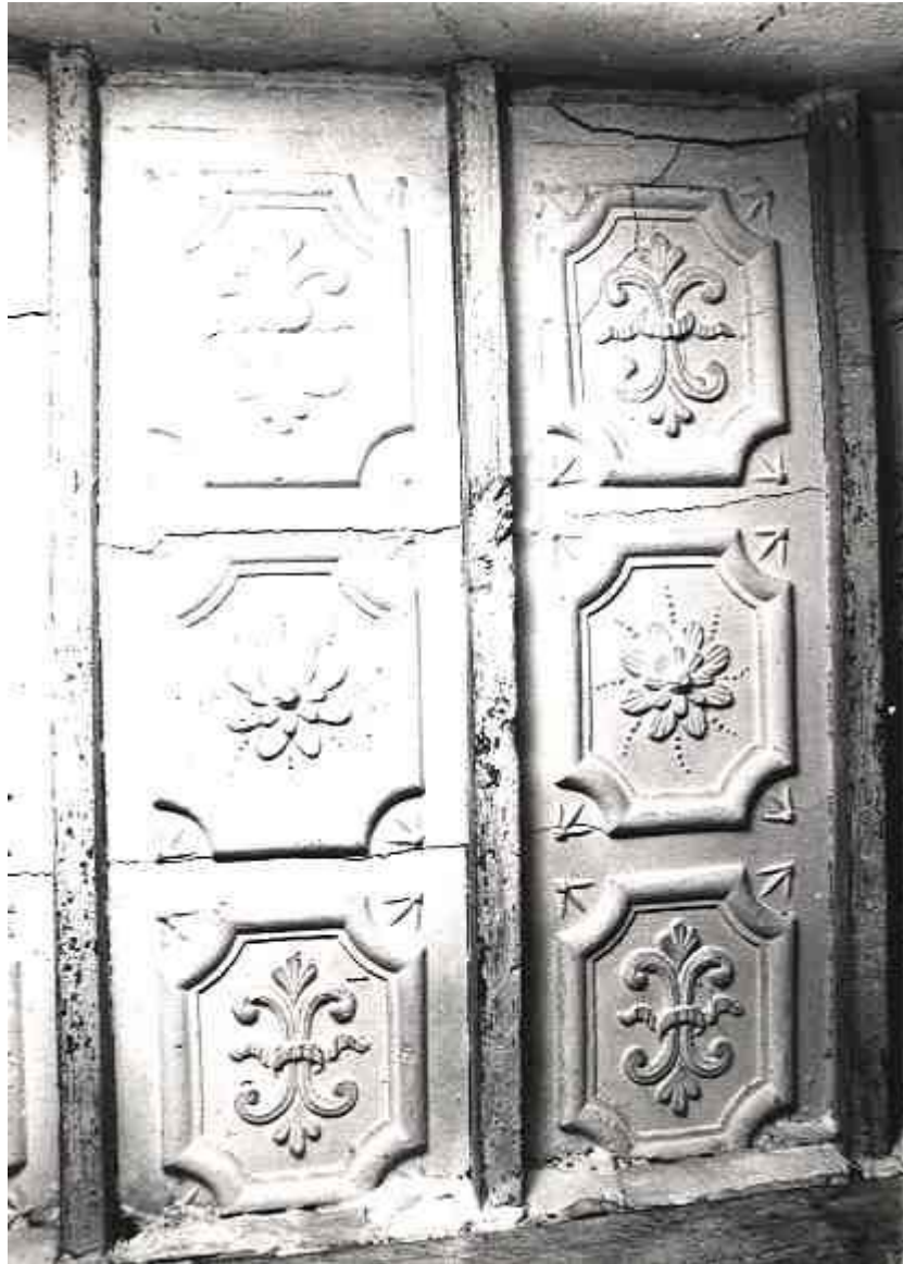
A typical gypsum ceiling (Asti)
