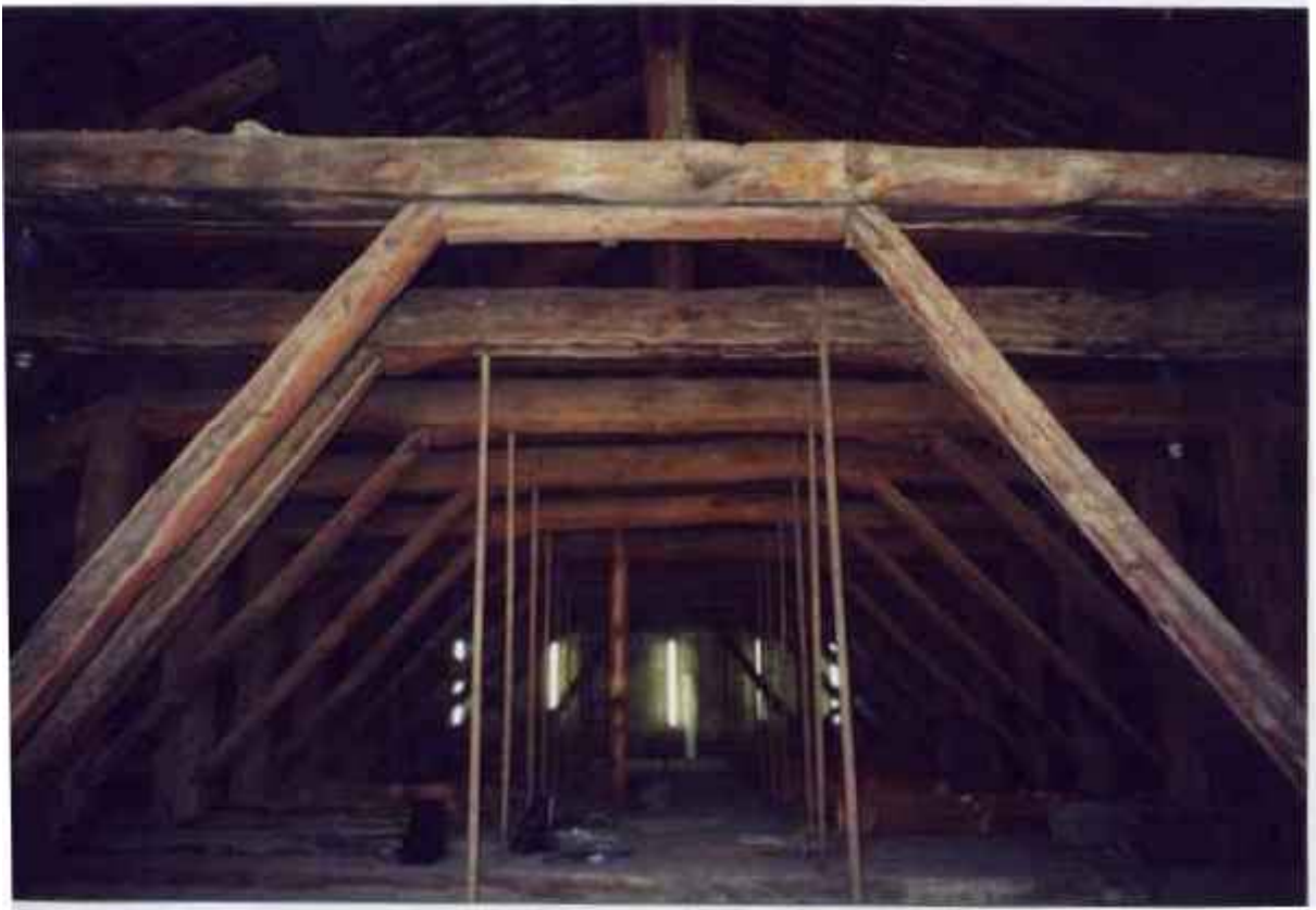
A prospective view of the wooden trusses installed above the central hall of Palazzo Madama in Turin
