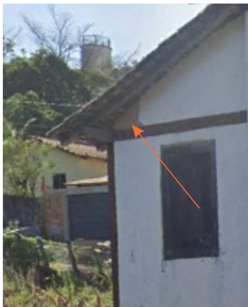
Decay: Delamination Possible Causes: Excess moisture; Incompatible materials; Rapid drying; Poor adhesion between the wall plaster layers; Structural movement; Incorrect mix composition Location: plaster applied under the roof
