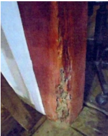
Decay: Wood-boring insects Possible Causes: Use of untreated or unprotected wood; Lack of preventive chemical treatment; Wood in direct contact with soil or damp masonry; High wood moisture content; Cracks or openings allowing insect entry; Warm and humid environments favorable to insect activity Location: Door jamb
