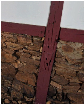
Decay: Wood splitting Possible Causes: Nail penetration causing localized stress and splitting along the wood grain. Location: Pillar
