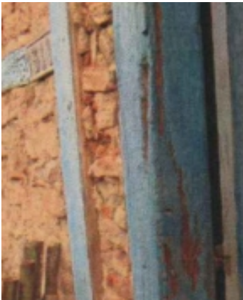
Decay: Wood-cracks Possible Causes: Loss of moisture causing contraction; Rapid or uneven drying; Internal stresses in the wood grain; Natural wood defects; Expansion and contraction cycles; Use of green wood; Mechanical stress or overloading; Aging and long-term weathering Location: Jamb
