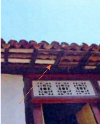
Decay: Wood-decaying fungi Possible Causes: Persistent moisture infiltration; Water trapped between tiles and wood; Failure of protective coatings. Location: Roof eaves
