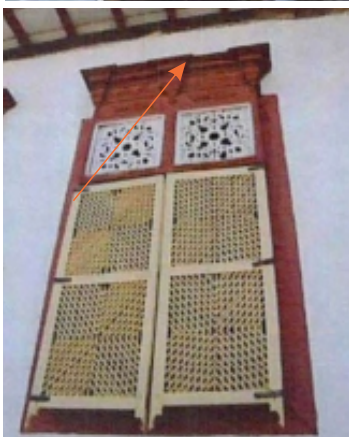
Decay: Soiling Possible Causes: Dirt from the ground or wall surfaces; Air pollution and vehicle emissions; Condensation attracting airborne particles; Bird droppings or insect activity; Accumulation in textured or rough window frames Location: Gelosia window
