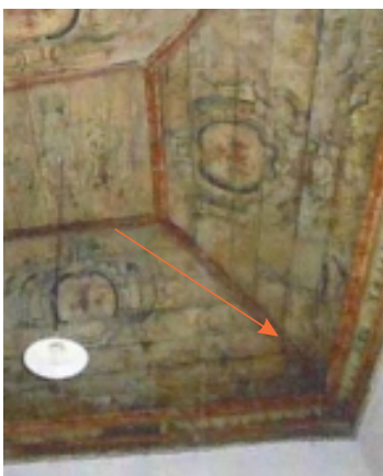
Decay: Mold Possible Causes: High indoor humidity levels; Poor ventilation in the room; Roof leaks allowing moisture to reach the wood; Condensation forming on the wood surface; Lack of protective coating or sealant on the wood; Thermal bridges causing localized dampness; Organic dust accumulation acting as a food source for mold; Inadequate insulation leading to temperature differences and moisture buildup Location: gamela ceiling
