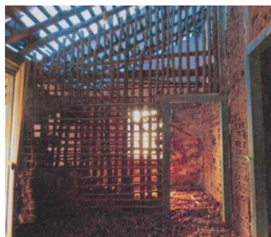
Total or partial reconstruction of wood locking and clay filling were used in the wattle and daub walls
