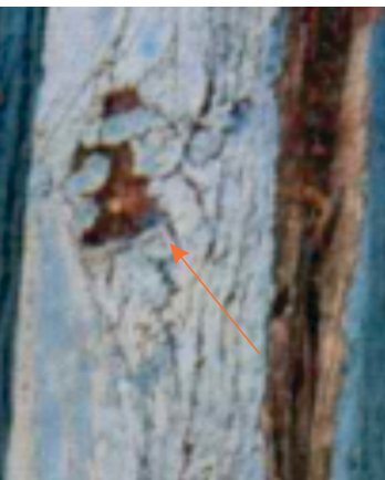
Decay: Craquelé in Paint Possible Causes: Wood movement due to humidity changes ; Application of paint over an unstable or dirty surface; Incompatible paint layers; Aged or degraded wood under the paint; Painting over a surface with residual moisture; Excessive paint thickness or poor layering; Sun and weather exposure causing thermal stress; Use of low-quality or expired paint Location: Jamb
