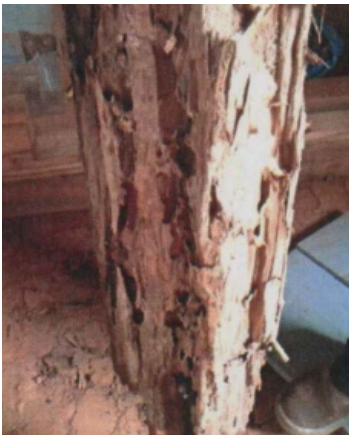
Decay: Wood-boring insects Possible Causes: Use of untreated or unprotected wood; Lack of preventive chemical treatment; Wood in direct contact with soil or damp masonry; High wood moisture content; Cracks or openings allowing insect entry; Warm and humid environments favorable to insect activity Location: Pillar
