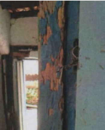
Decay: Wood-boring insects Possible Causes: Use of untreated or unprotected wood; Lack of preventive chemical treatment; Wood in direct contact with soil or damp masonry; Cracks or openings allowing insect entry; Warm and humid environments favorable to insect activity Location: Jamb
