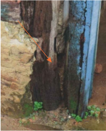
Decay: Wood-decaying fungi Possible Causes: Persistent moisture infiltration; Water trapped between paint layers and wood; Failure of protective coatings. Location: Pillar
