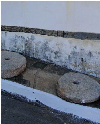
Decay: Rising damp Possible Causes: Degraded or failed damp-proof barrier; Capillary action drawing moisture from the soil into the masonry; Soil in direct contact with stone walls without protection; Use of impermeable plasters or coatings trapping moisture inside; Water accumulation around the foundation due drainage failures Location: exterior wall
