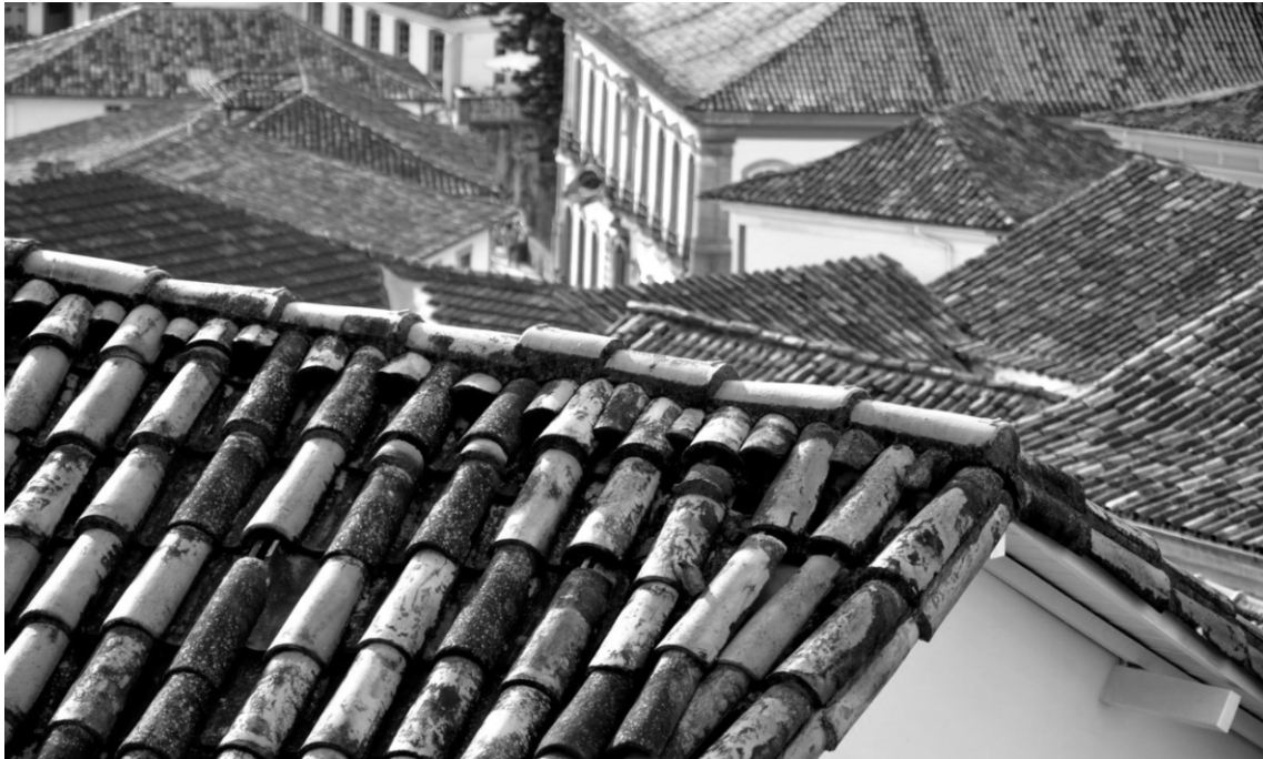
Figure 58 – Roofs in a colonial city in Brazil [Source: Photo available at Freeimages.com]
