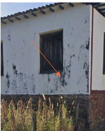
Decay: Moisture darkening Possible Causes: Water infiltration from rain or leaks; Rising damp from the ground; Lack of protective overhangs or drainage; Use of non-breathable surface coatings; Hair cracks allowing moisture ingress Location: exterior wall painting
