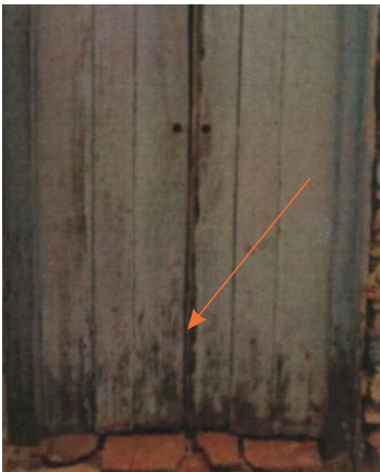
Decay: Wood-decaying fungi Possible Causes: Persistent moisture infiltration; Water trapped between paint layers and wood; Failure of protective coatings. Location: Door
