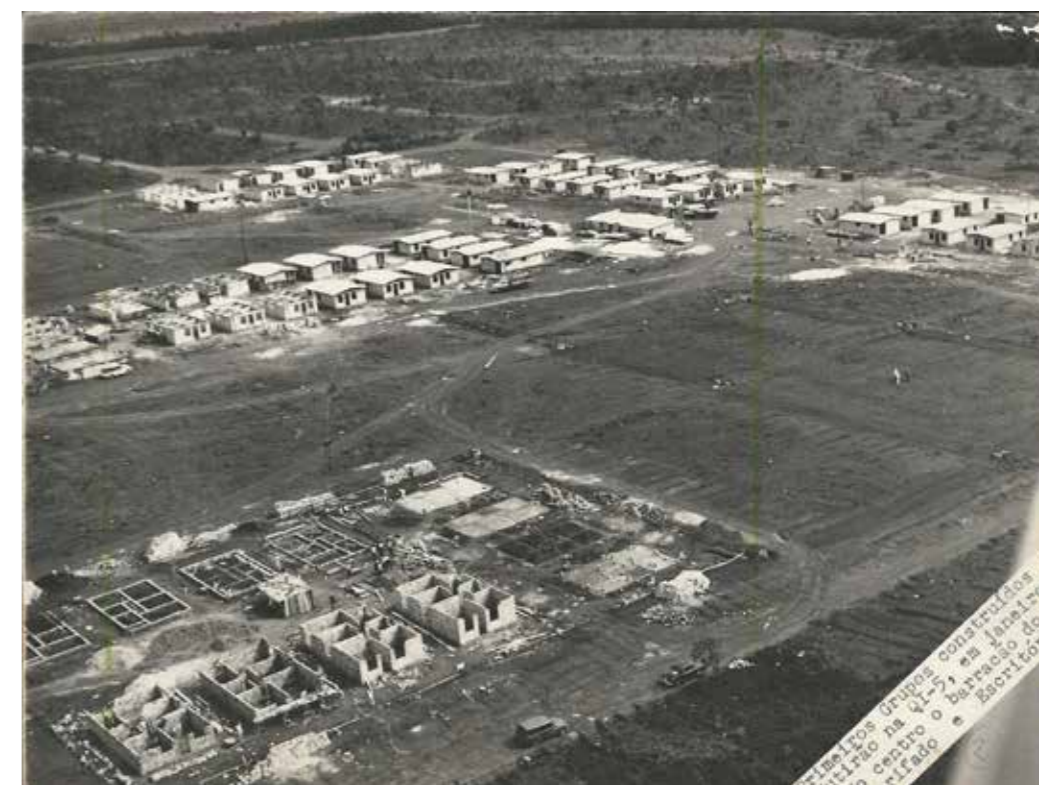
Figure 14: Ariel view of the construction of one of the first block of Guar4 I. Source: Jornal do Guar4, 2021
