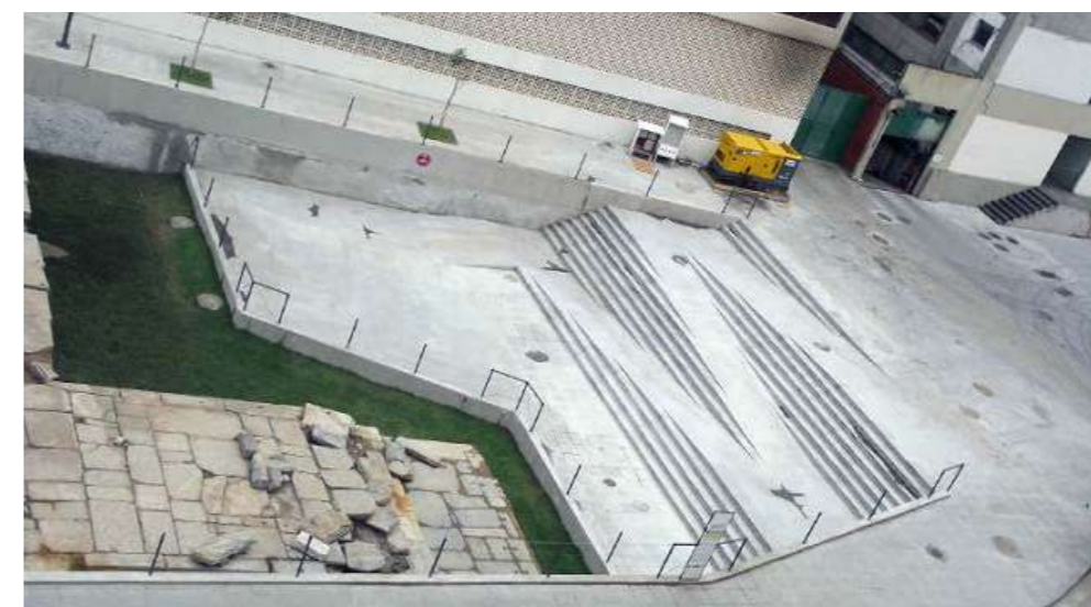
Fig. 77 Stairs, access ramps, and observation point for the public. Source Tânia Andrade Lima
