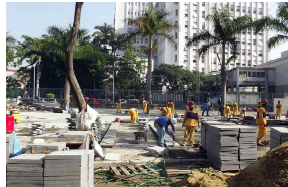
Fig. 75 Laying of the new pavement with granite slabs. Source Tânia Andrade Lima
