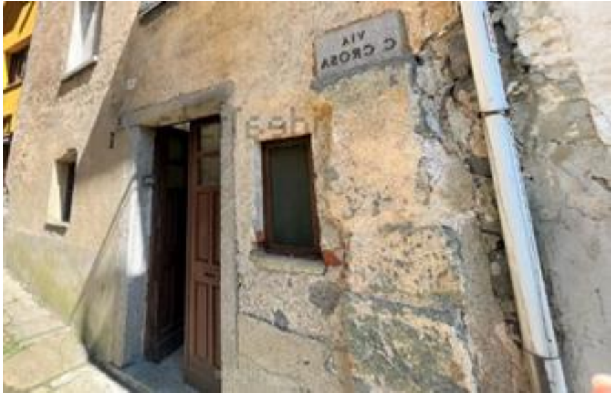
Figure 17 Damaged buildings of Rosazza
