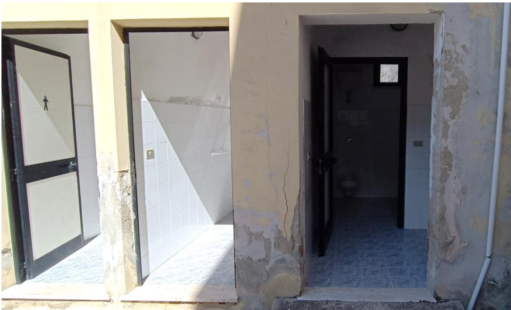
Figure 140- External plaster degradation (US2).
