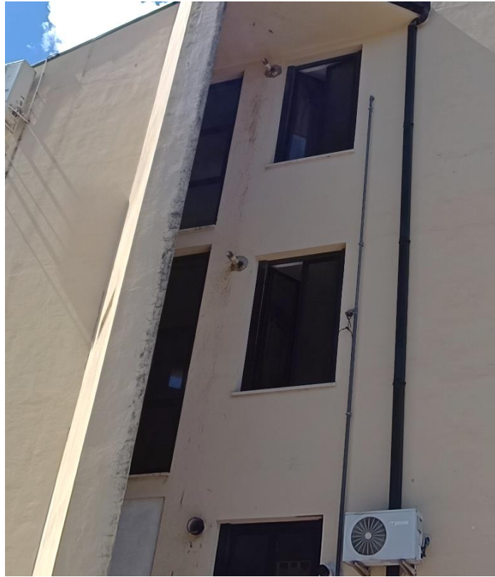
Figure 3 -The partition is experiencing rebar cover expulsion (US1).
