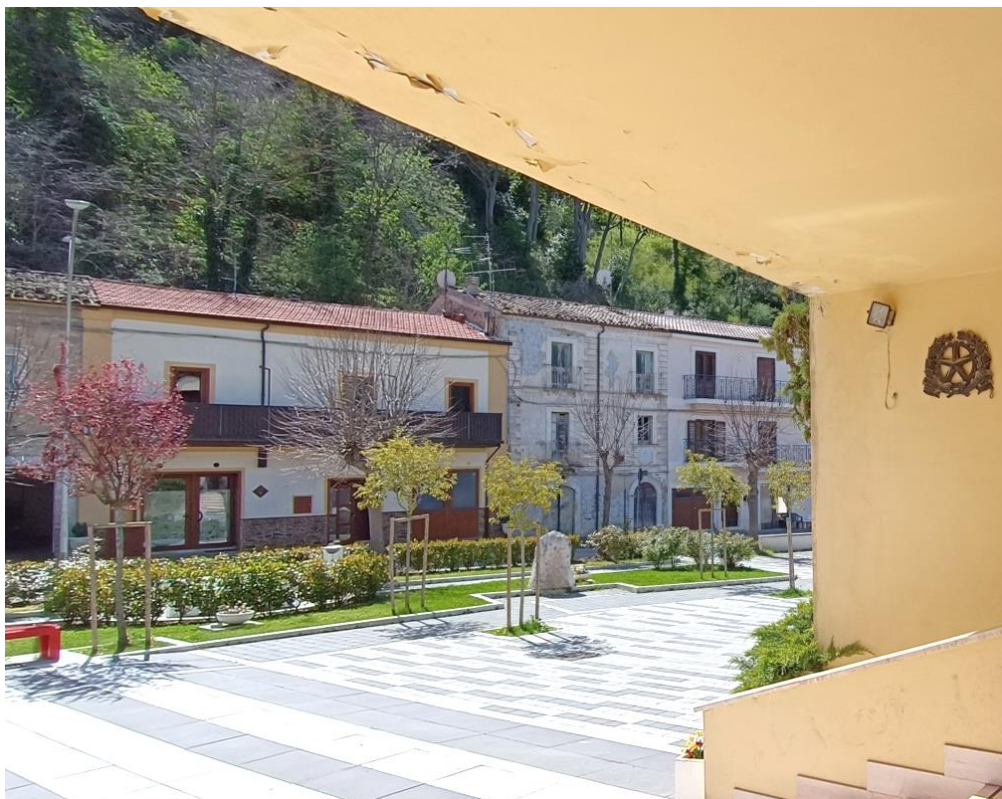
Figure 144 - material degradation on the underside of the balcony (US1)
