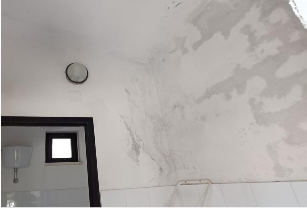
Figure 141- Internal plaster degradation (US2).
