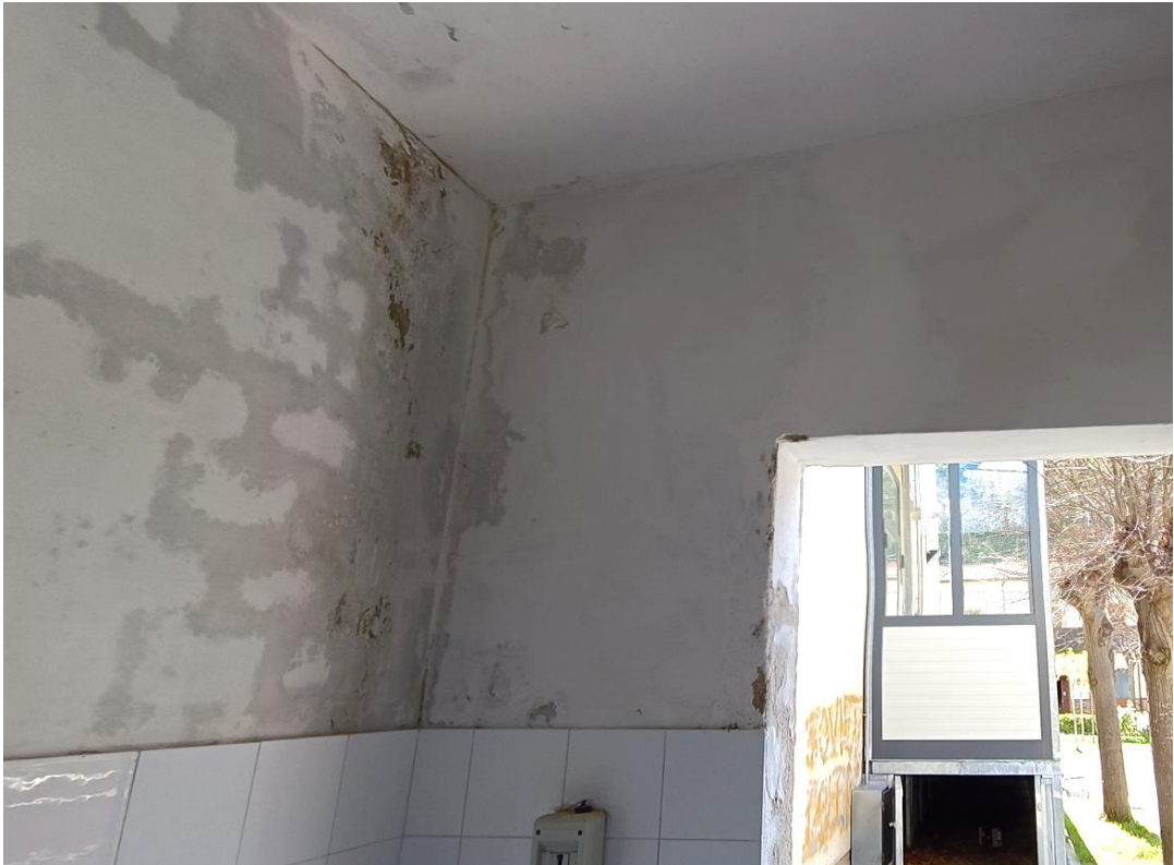
Figure 142 - Internal plaster degradation (US2).
