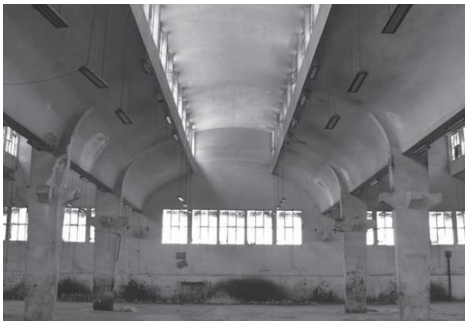
Fig.5.21. The new bleach facility for fabrics, with an inside perspective of the overhanging shelled roofing, El-Shirka El-Ahliyya. (The Alexandria and Mediterranean Research Center)
