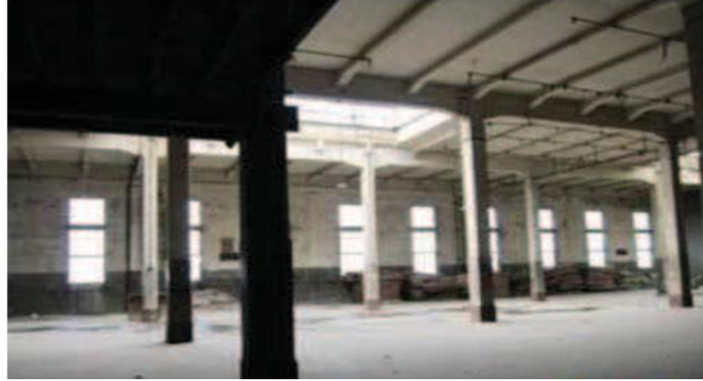
Fig.6.8. Present condition within the cotton warehouse of Makbas El Tarekk (Author & ANPIEMED)
