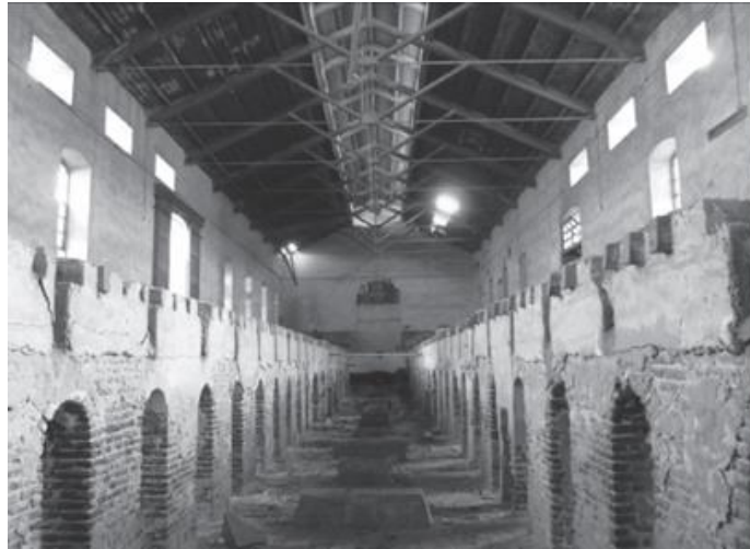
Fig.4.23. The internal perspective of the main ginning hall at Salvago Ginning Plant showing the framework that supported the building before the main floor was demolished. (Bibliotheca Alexandrina)
