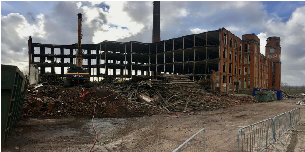
Fig.3.3. The abandoned Hartford Mill industrial structure near Oldham, United Kingdom,
