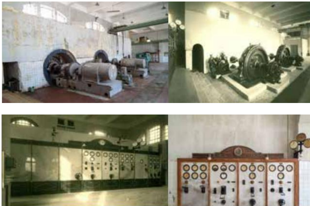
Fig.4.46. El Faiyum Energy Station showing the old and the modern turbines. (Explore Fayoum, https://fayoumegypt.com/explore-fayoum-with-fayoumer/ )
