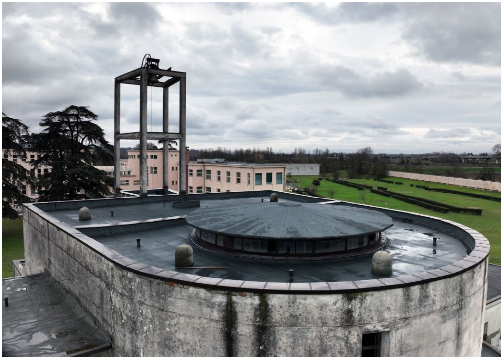
Fig. 20. Present condition of the roof. Source: Team DIRECT
