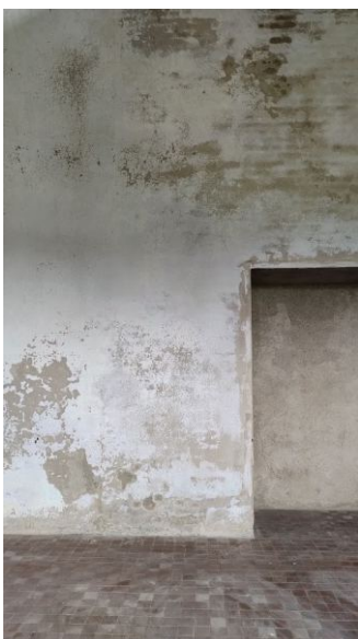
Fig. 45, 46, 47, 48 (from left to right). Degradation inside next to the confessional (fig. 45). Degradation of the ambulatory’s roof (fig. 46). Degradation of the window at the morgue block (fig. 47). Degradation of a wall in the central nave (fig. 48). Source: By the authors 2024.
