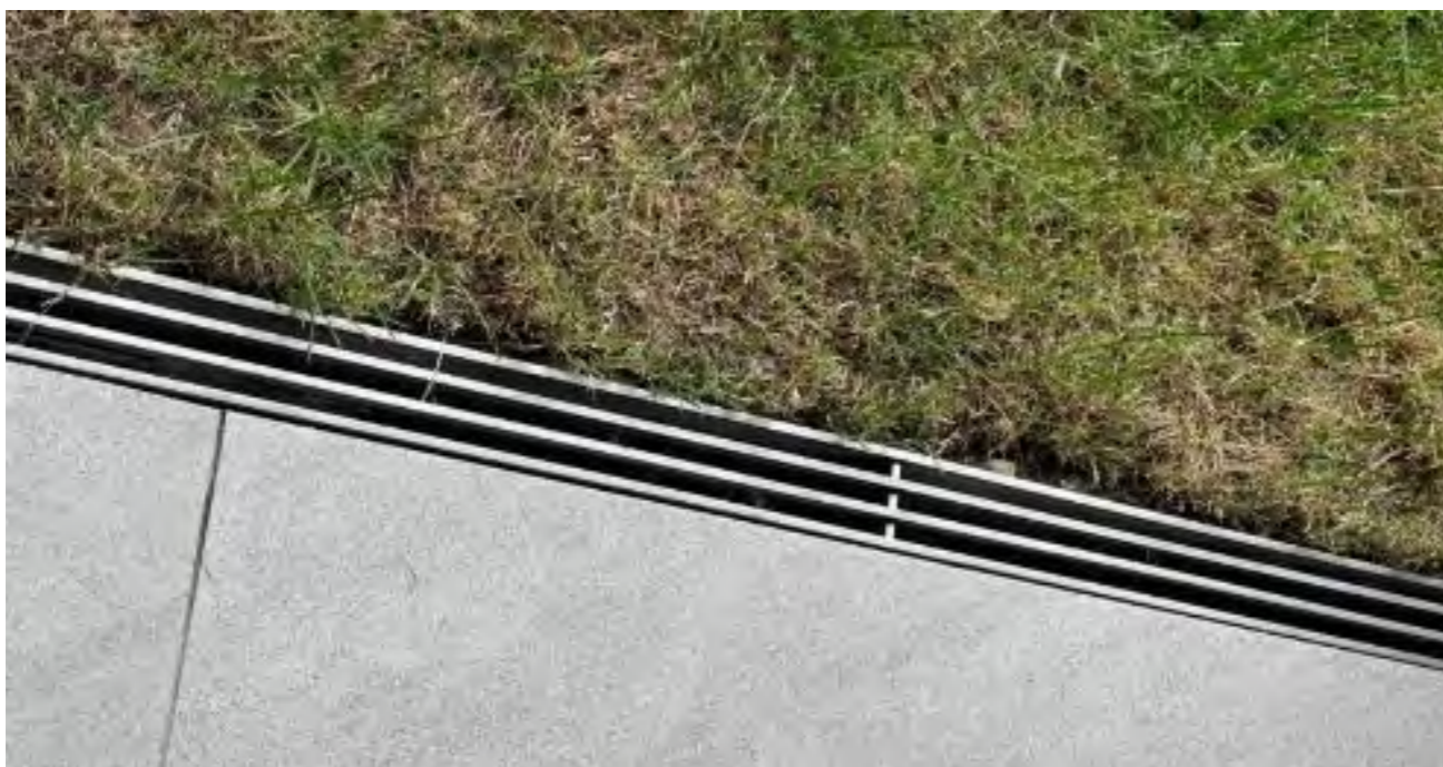
Figure 71 : Integrated Management Building ground water return system
