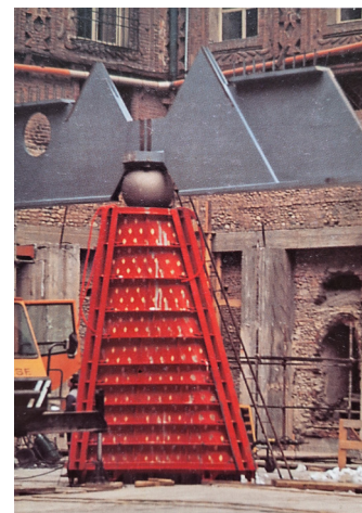
Fig. 3.13. A detail of one of the new pillars of the underground hall designed by Bruno. Source: Mastropietro, Oltre il Restauro , 229.
