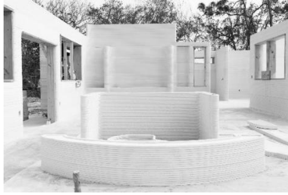
Image 4 Apis Cor's 3D-printed concrete walls for a residential house in Melbourne, FL. Source: (Apis Cor, a Manufacturer of Construction 3D Printing Robots, Announces Strategic Investment by D.R. Horton, 2024).
