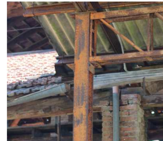
Image 73 Corrosion on structural column
