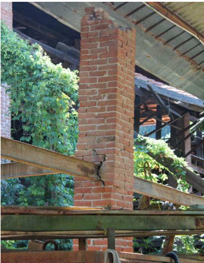
Image 84 Addition of a steel beam that expands and contracts affecting brick column Source: Photo by the authors, 2024
