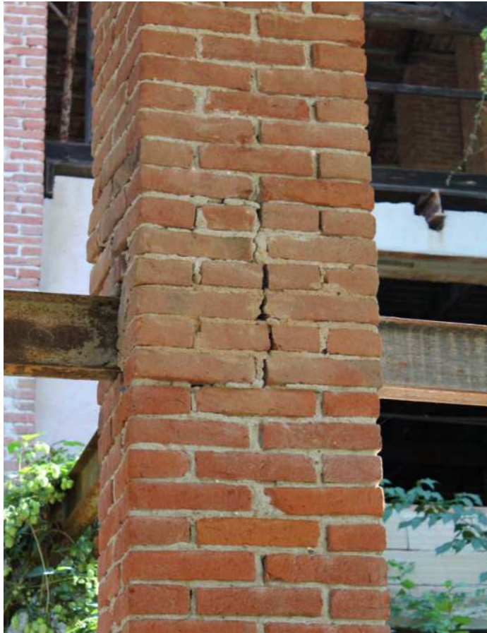
Image 82 Addition of a steel beam that expands and contracts affecting brick column Source: Photo by the authors, 2024
