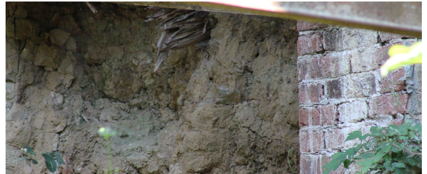
Image 86 Sun dried bricks and kiln fired bricks creating cracks between each Source: Photo by the authors, 2024
