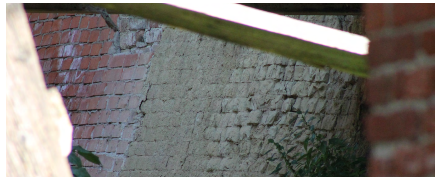
Image 87 Sun dried bricks and kiln fired bricks creating cracks between each Source: Photo by the authors, 2024
