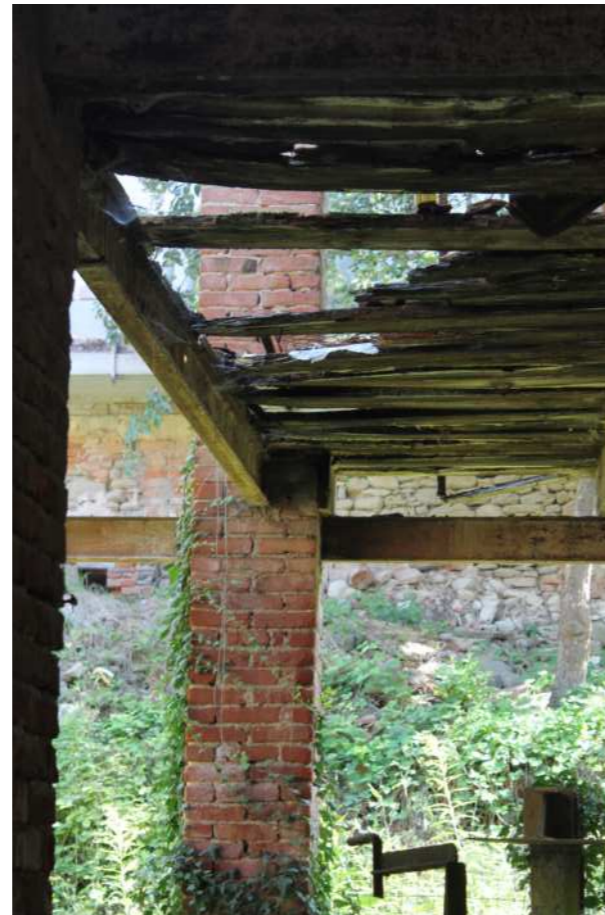
Image 72 Wooden roof deterioration Source: Photo by the authors, 2024
