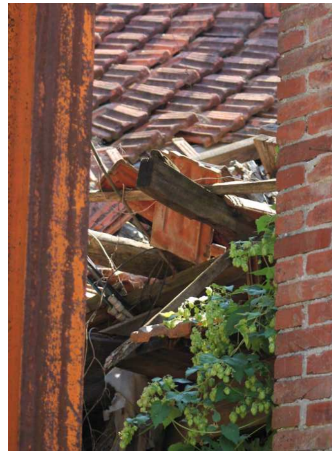
Image 71 Wooden Roof deterioration Source: Photo by the authors, 2024
