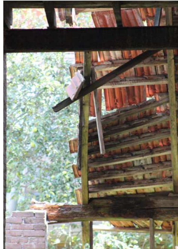
Image 70 Cracking wooden floor Source: Photo by the authors, 2024
