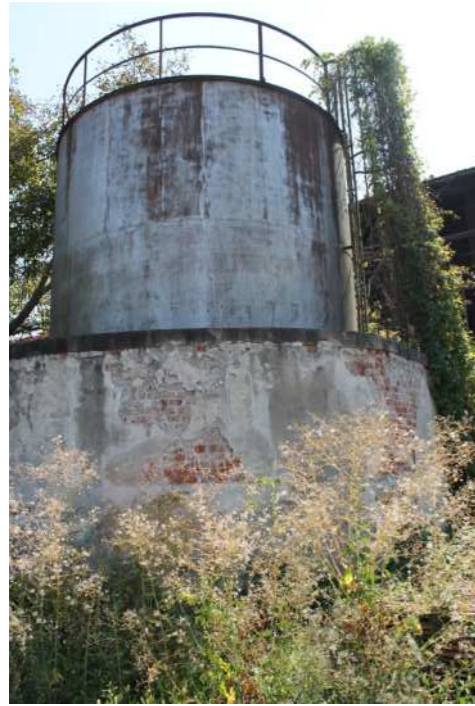
Image 88 Corrosion of the gas-oil tank Source: Photo by the authors, 2024
