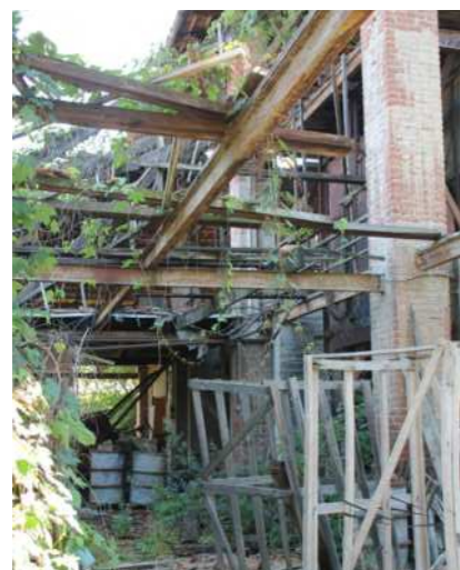
Image 50 Collapsed floor from the lateral naves Source: Photo by the authors, 2024
