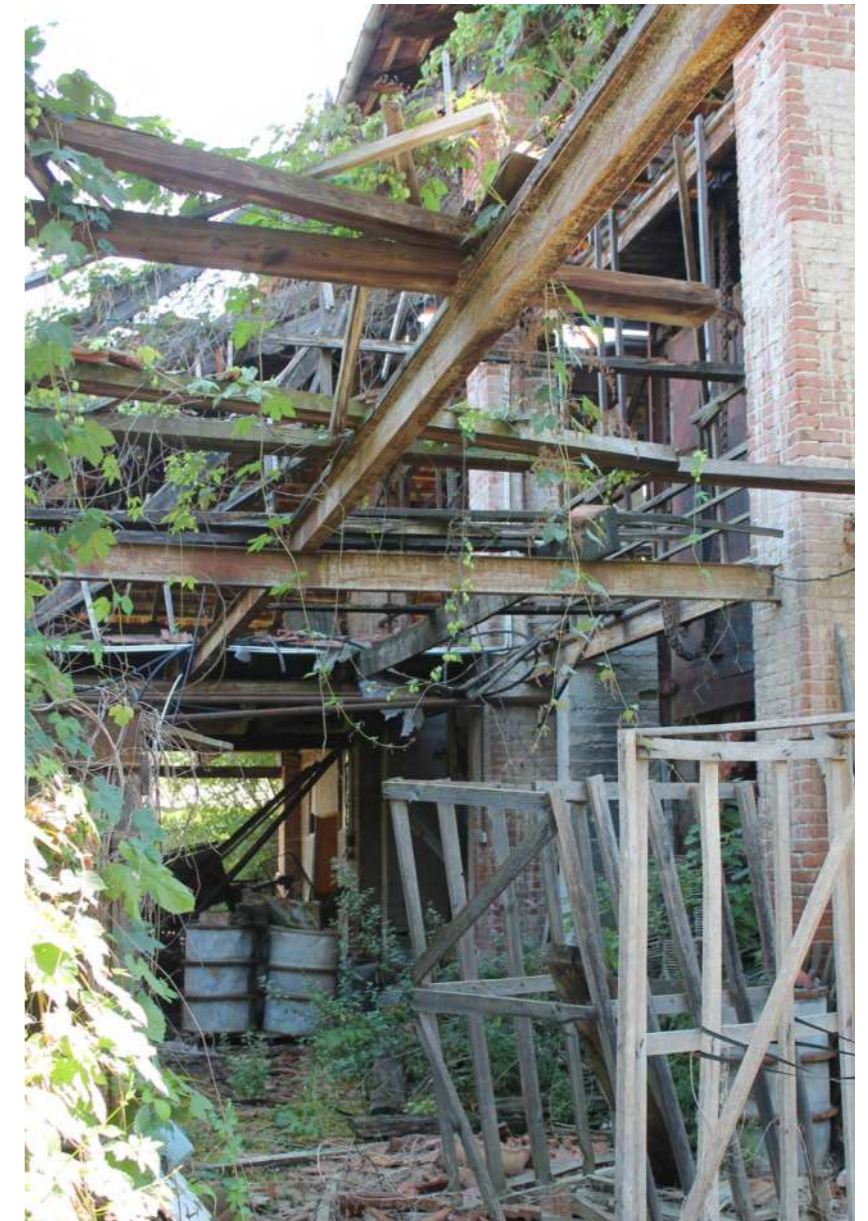
Image 76 Bending beam supporting what used to be a wooden floor Source: Photo by the author
