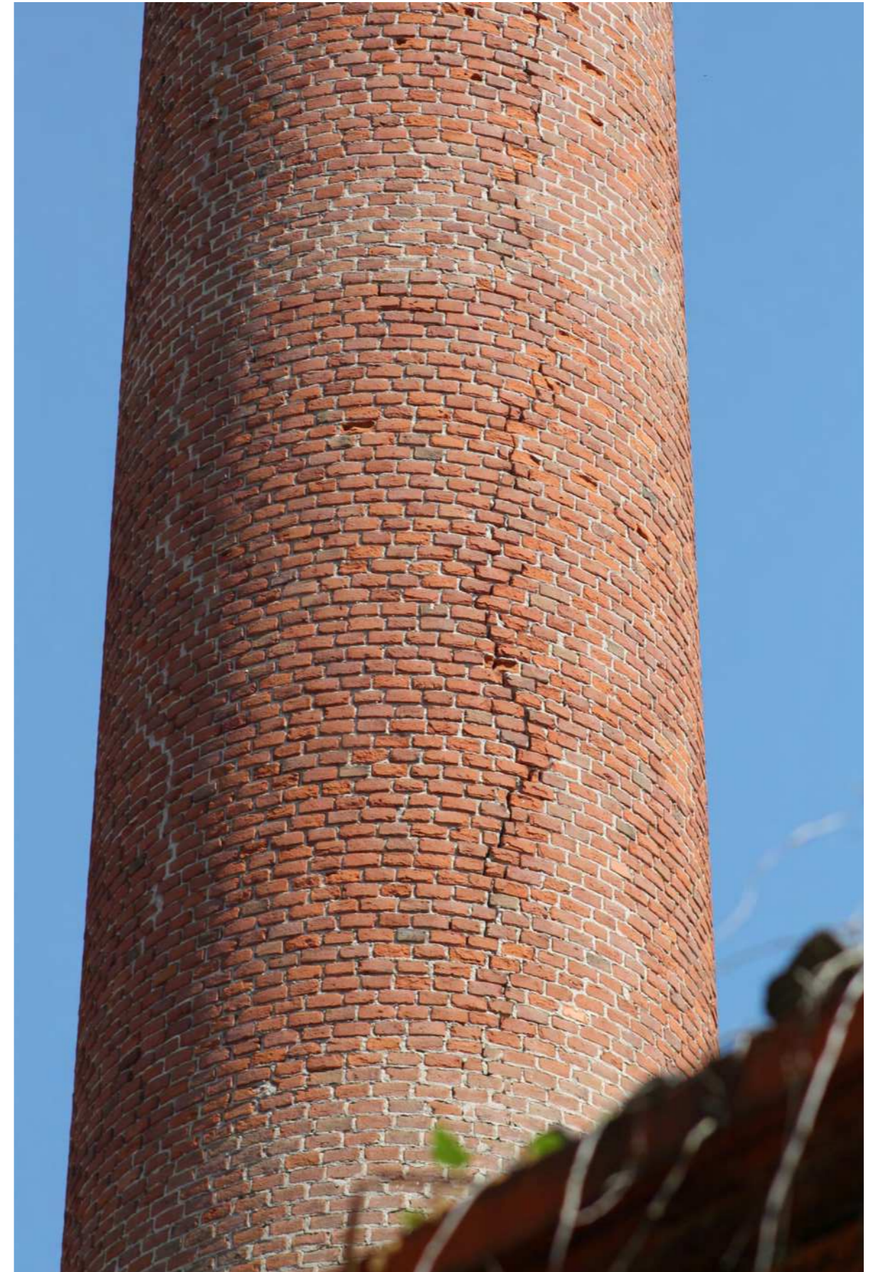
Image 69 Cracks in the chimney Source: Photo by the authors, 2024
