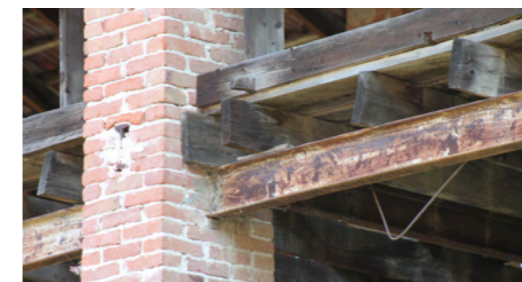
Image 75 Expansion of beam and cracking of brick column
