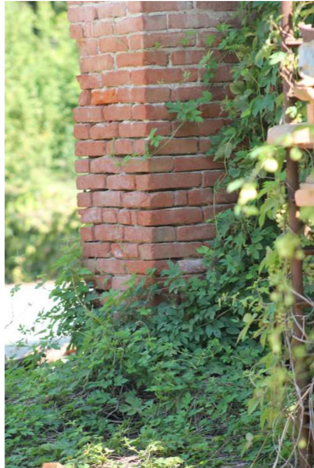
Image 62 Column with rising damp, brick color intensification Source: Photo by the authors, 2024
