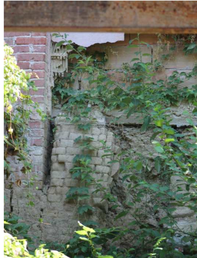
Image 83 Sun dried bricks and kiln fired bricks creating cracks between each Source: Photo by the authors, 2024
