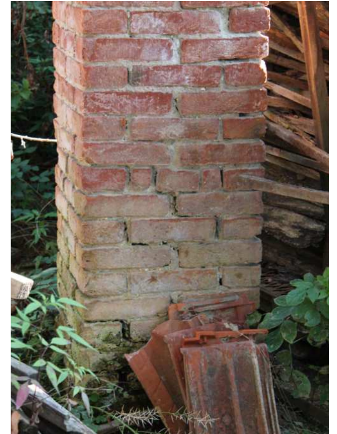
Image 65 Efflorescence, salt deposits Source: Photo by the authors, 2024
