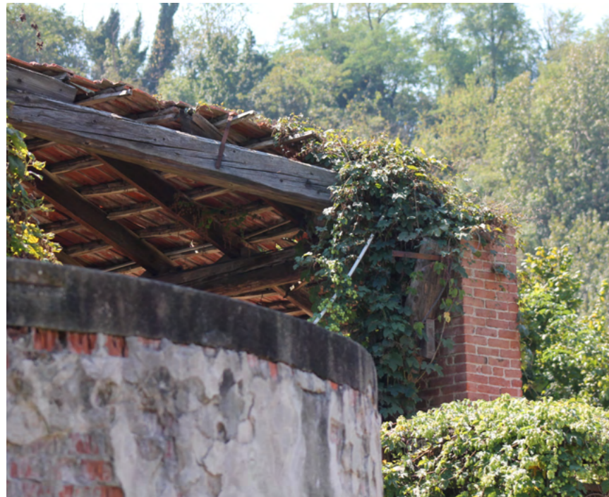
Image 90 Biological growth on brick column and wooden roof Source: Photo by the authors, 2024
