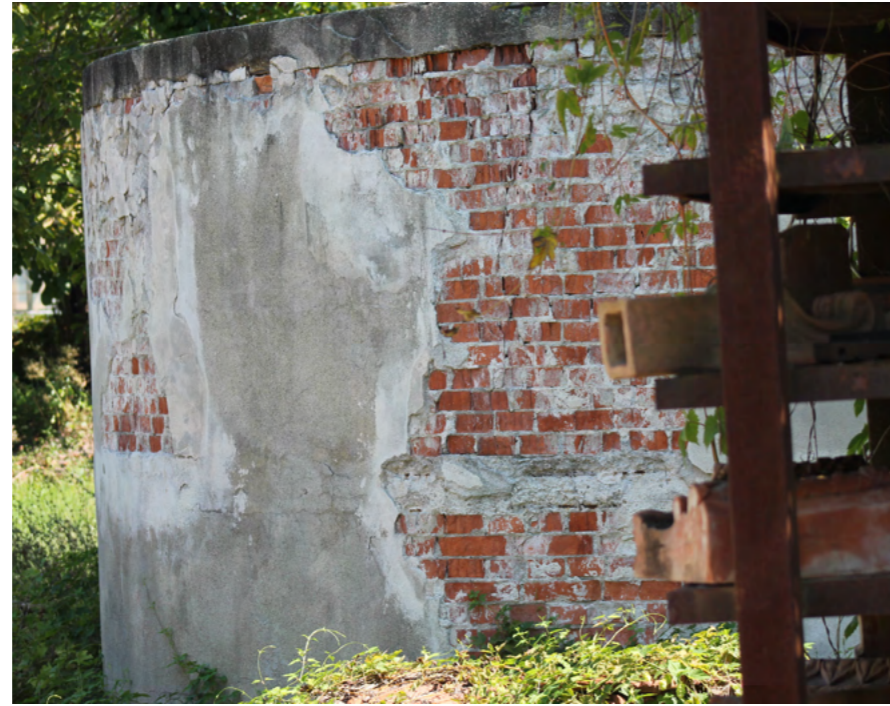
Image 89 Detachment of plaster due to rising damp Source: Photo by the authors, 2024
