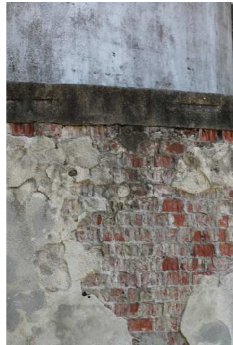
Image 91 Detachment of plaster due to rising damp Source: Photo by the authors, 2024
