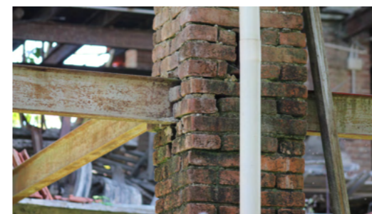
Image 74 Expansion of beam and cracking of brick column
