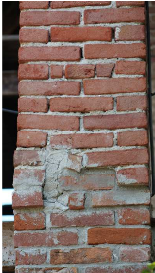
Image 67 Expansion of the bricks leading to cracks Source: Photo by the authors, 2024
