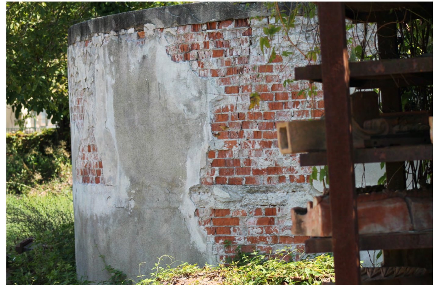
Image 63 Detachment of plaster and paint Source: Photo by the authors, 2024
