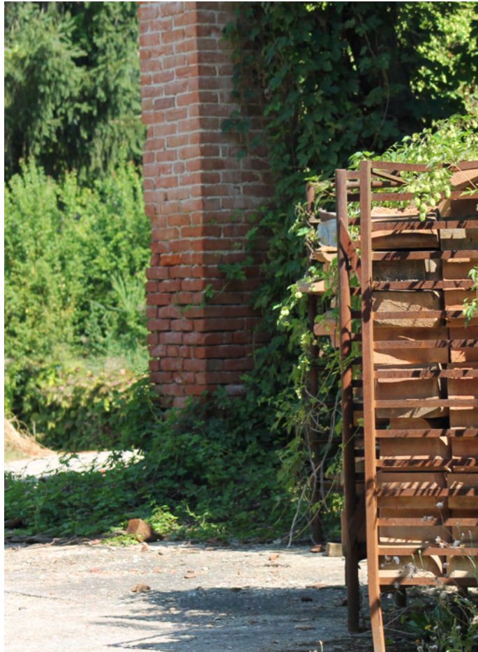
Image 61 Column with rising damp, brick color intensification Source: Photo by the authors, 2024
