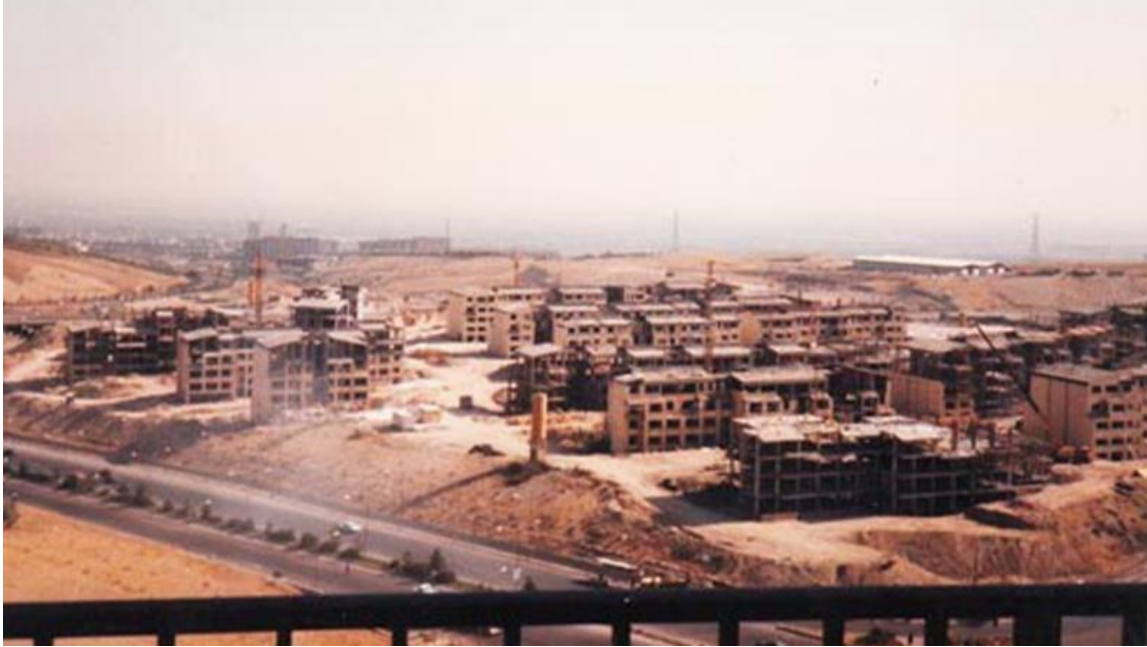
Figure 34 : This image depicts the initial stages of construction in Shahrak-e-Gharb, highlighting the introduction of modern urban planning principles in the neighborhood. The emphasis on structured layouts and villa designs reflects Western architectural influences. (Melkonline, 2021)
