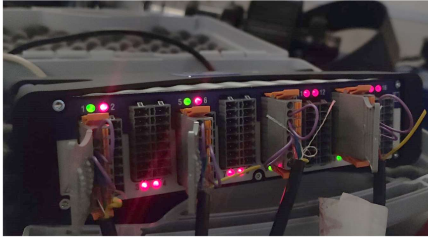
Figure 28: Connection to the HBM acquisition board.
