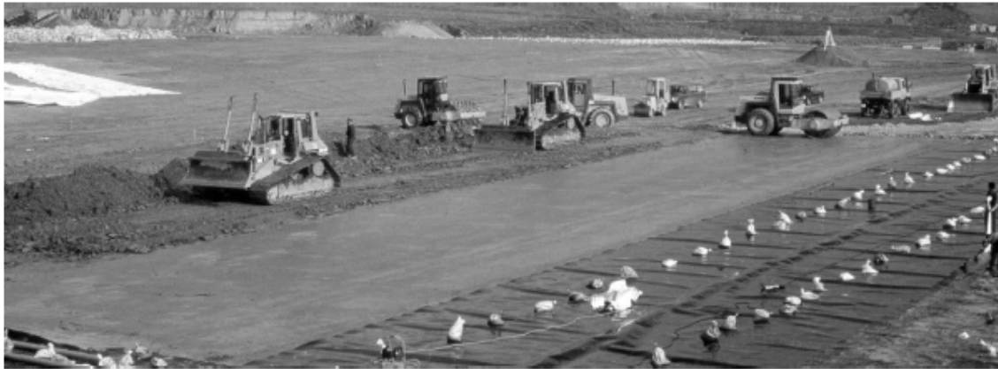
Figure 3.15 Watering, Sheep-foot compacting, levelling, smooth compacting (typical for two layers) - Source 3-K-VON-MAUBEUGE-Naue
