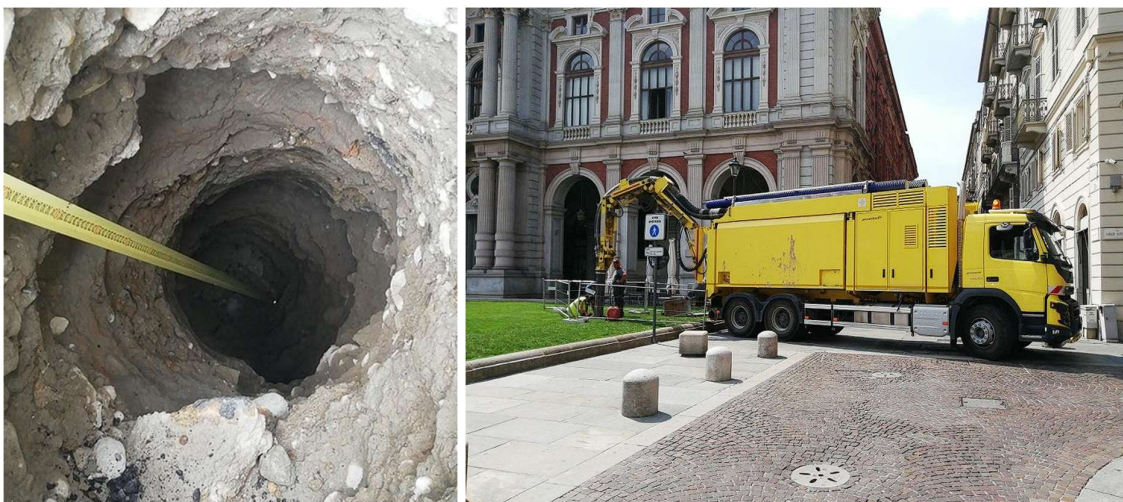
Figure 4.13. From left to right: inside of a borehole drilling and the survey activity (Infratrasporti.To S.r.l, 2023)
