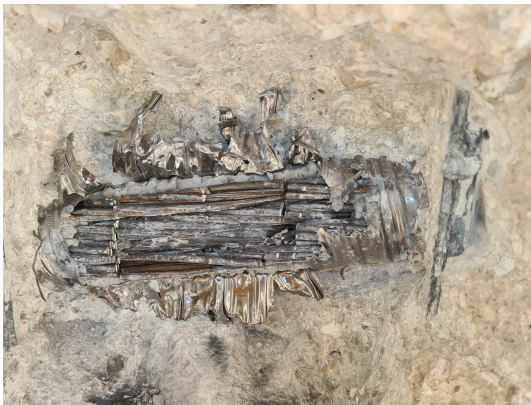
(c) Detail of exposed strands on Cerqueta Bridge.
