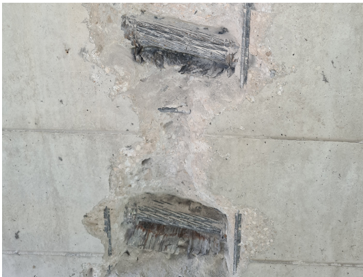
(a) Opened section showing two cable cut locations on Cerqueta Bridge.
