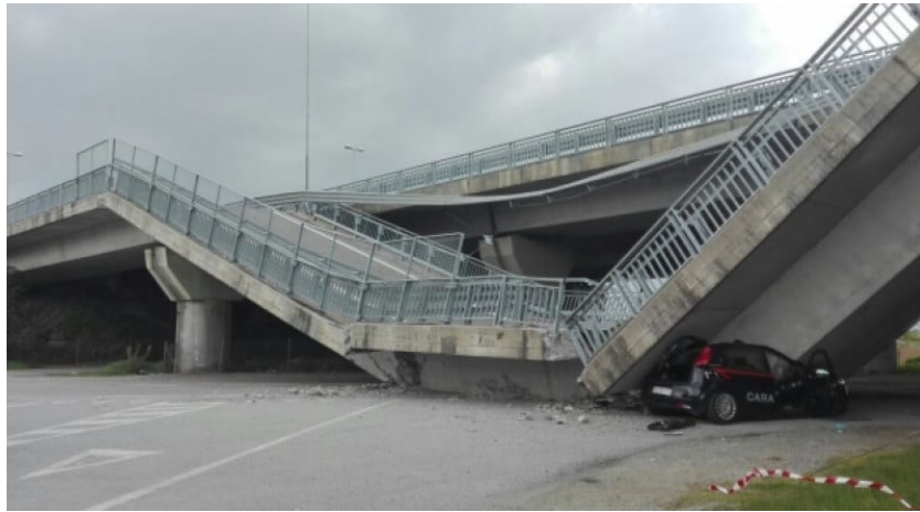
Figure 1.2: The collapse of the La Reale viaduct in Fossano, Italy, highlighting the consequences of wire corrosion and structural deficiencies.
