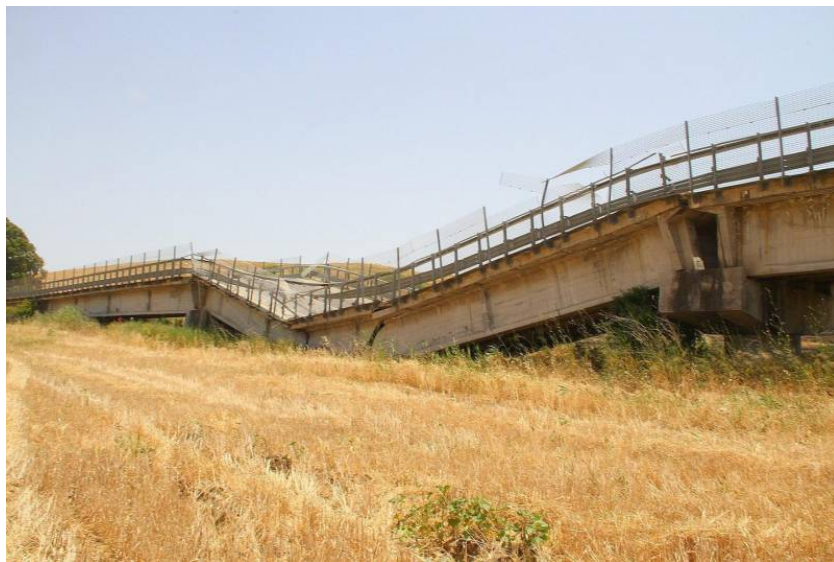
Figure 1.3: The partial collapse of the Petrulla viaduct in Agrigento, Italy, due to the failure of prestressed concrete beams.
