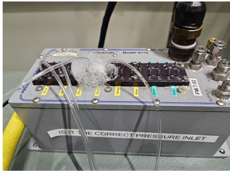
Figure 5.3: Example of a leak at the 9116 NetScanner
