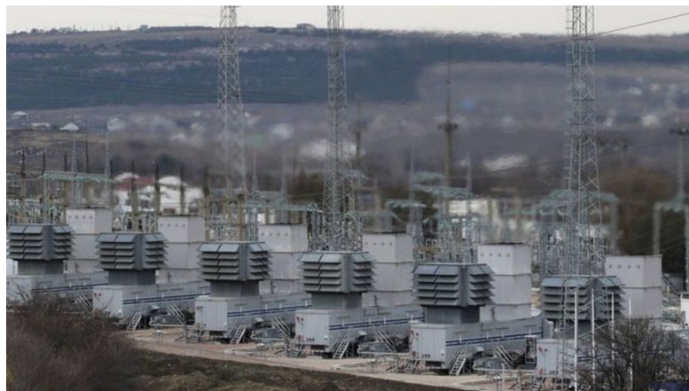
Figure 1.4: Western Ukraine’s Prykarpattiaoblenergo utility [6].
