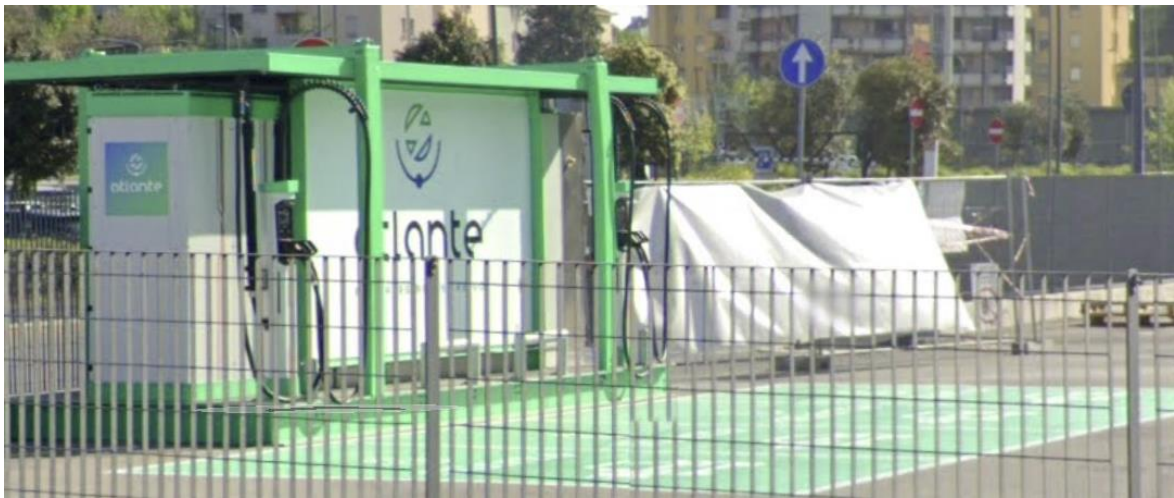
Figure 54: Atlante storage with connected EVs charging infrastructure.
