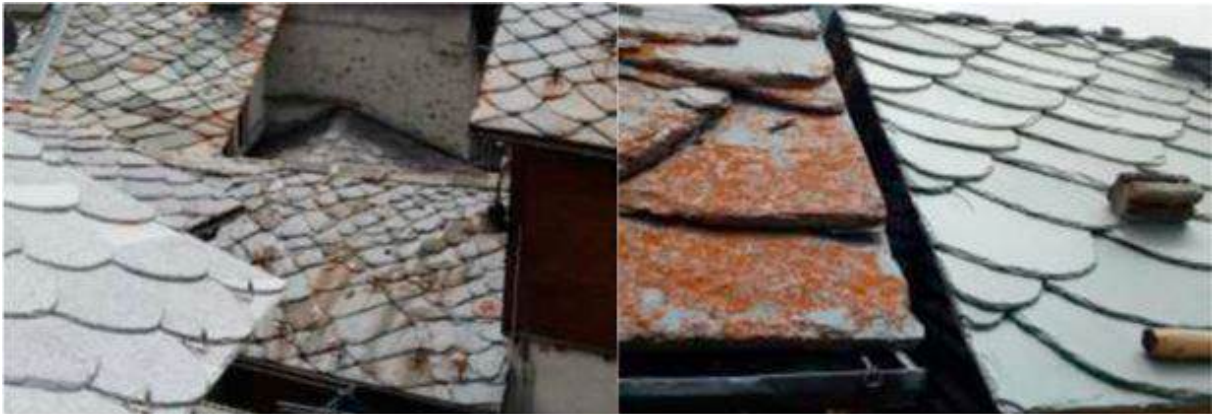
Figure 24. Porfiroide roofing near the new roofs of gneiss on the left and Quartzite on the right in Antagnod. Source: Journal of Building Engineering Elsevier
