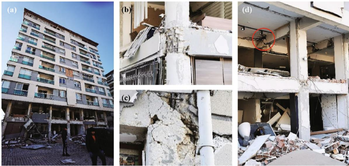
Figure 4: Example of a severely damaged building in Antakya (Wang et al., 2023, p 856)
