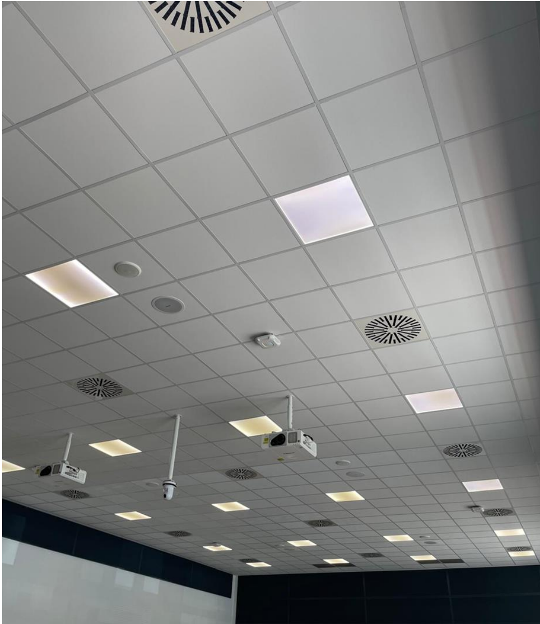
Figure 13: The ceiling view shows that there are 4 electrical lightings in each row.
