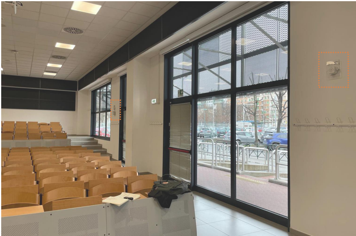
Figure 20: Sensors 2 and 22 mounted on the wall facing outside in classroom 1P.
