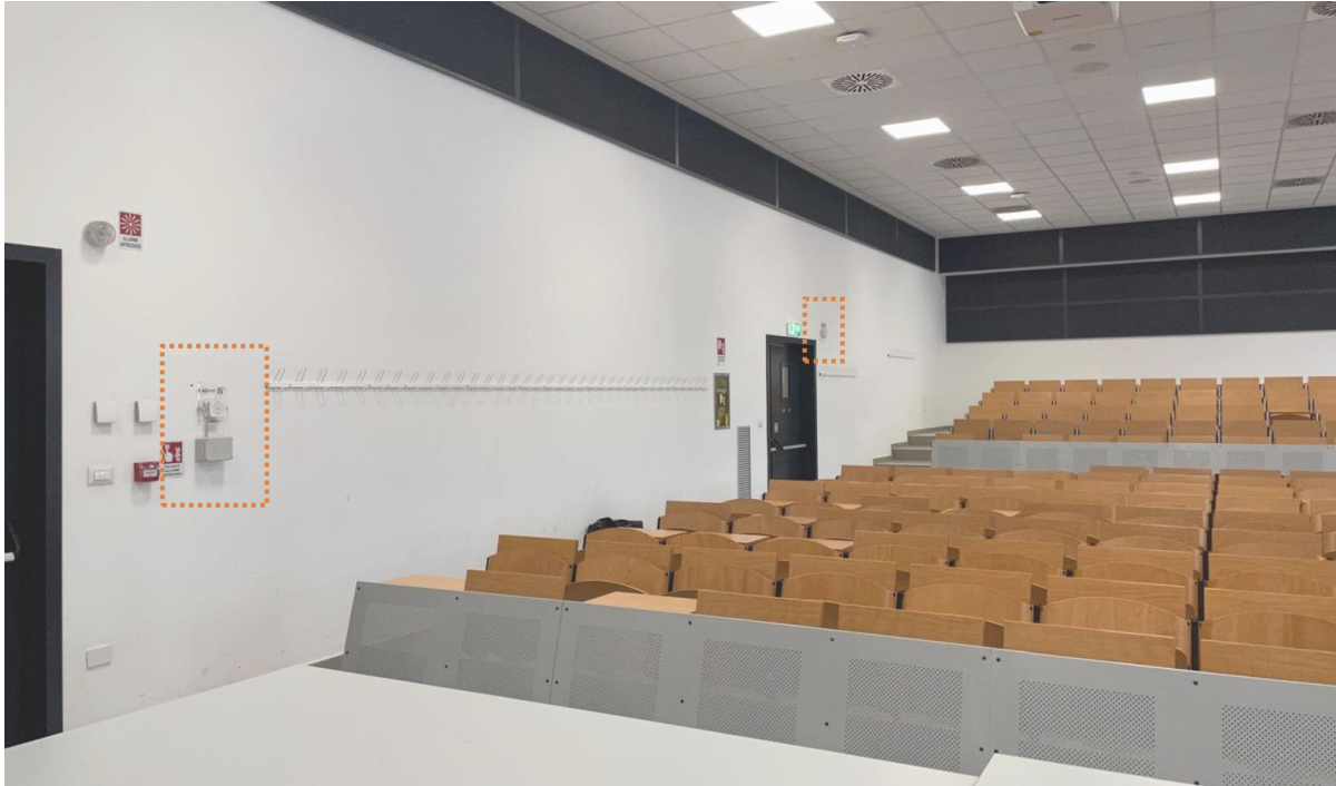
Figure 19: Sensors 1 and 21 mounted on the wall facing the interior corridor in classroom 1P.
