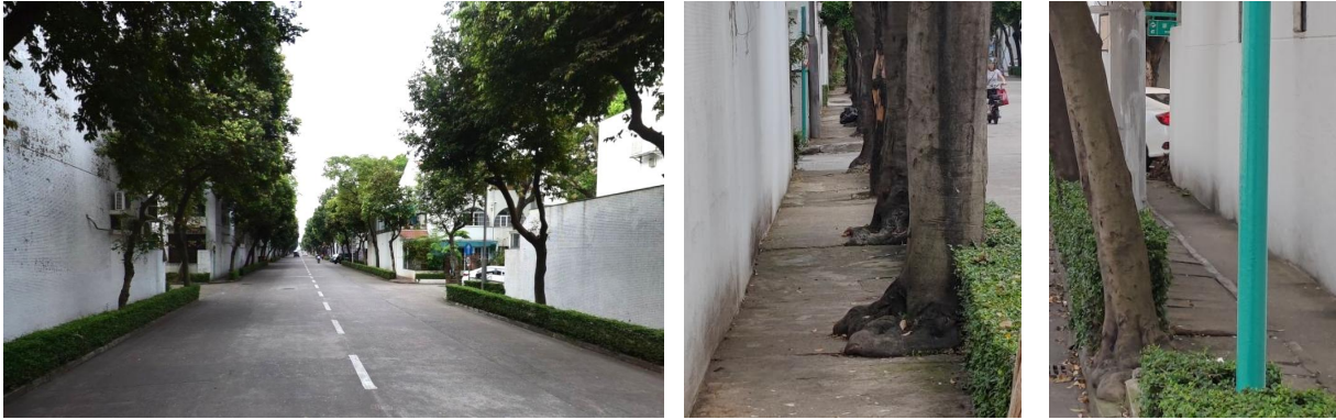
Figure 6-18: Footpaths current condition of Fuhua Road
