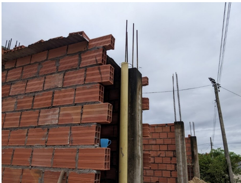
Figure 2: Photography - Industrialized Materials used in the construction of housing in rural areas - Acacias, Meta, 2022
