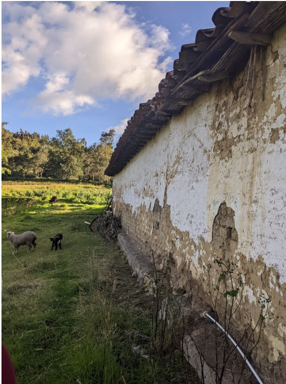
Figure 1: Photography – Traditional rural house wall construction with adobe block technology - Sogamoso, Boyacá, 2022
