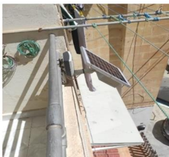
Figure 12 Sensors are to be installed at various locations, mostly within Gżira, to collect and compare data at different geographical points to identify the various pollutants. Handheld sensors (indicated as light blue on the map) will be provided to citizens who will be interested in participating in the data collection of pollutant measurements.
