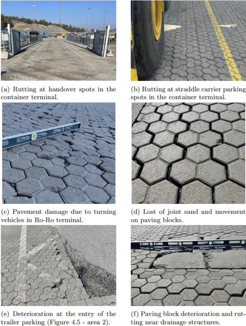
Figure 2.1.8: Damage in the port area (J. D. Rodriguez Millan, 2024)
