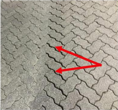
Figure 1.2.5: Example of surface failure in ICBP (Jamshidi et al., 2019)
