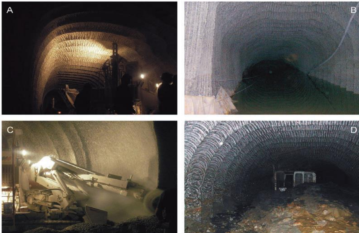
Figure 4 shows the drift before and after the sediment and water flow. Gypsum was being cut with a road header on February 15, 2005, just before the inrush; on February 16, 2005, the road header was nearly entirely covered by mud. On February 15, 2005, the water level stabilized at 139 meters above sea level. (Article in Zeitschrift für Geomorphologie Supplementary Issues · May 2010, Hypogene gypsum karst and sinkhole formation at Moncalvo (Asti, Italy)).
