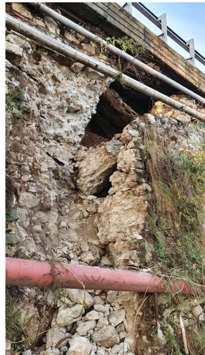
Figure 25. Damage on the retaining wall
