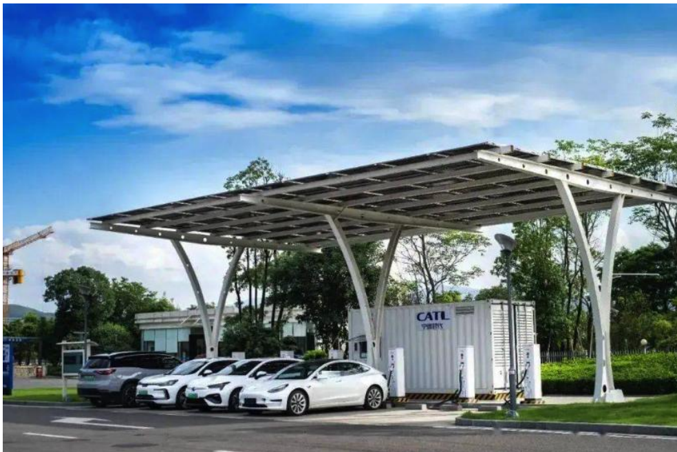
Figure 2.2.3 PV-integrated charging station
