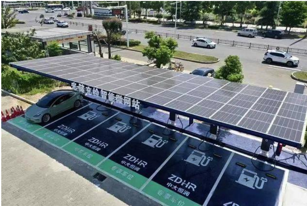
Figure 2.2.2 PV-integrated charging station
