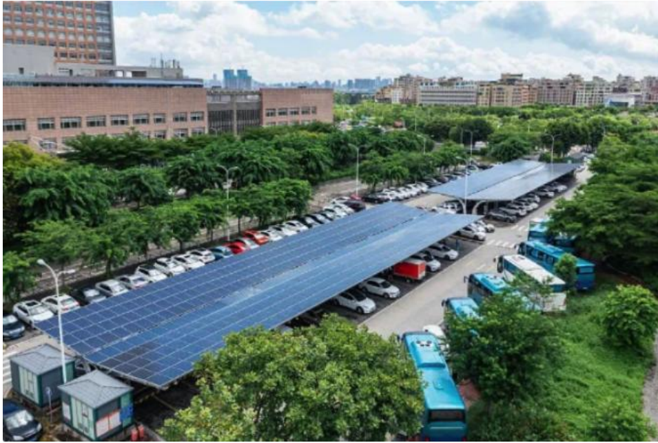
Figure 2.2.4 PV-integrated charging station
