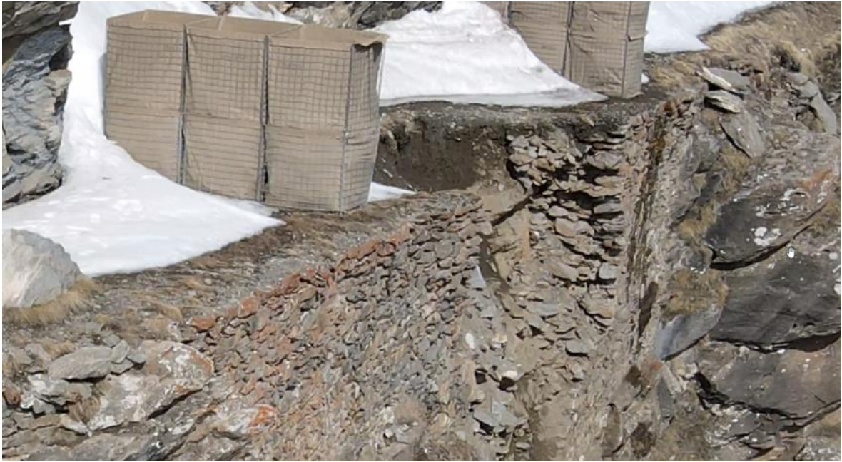
Figure 17 - Detail of big bags. In this image, the collapsed section of the wall is clearly visible (courtesy of Casale M.).
