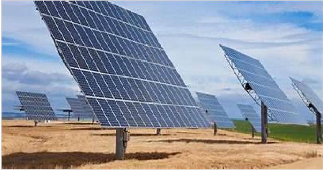
Figure 8. Photovoltaic solar panels
