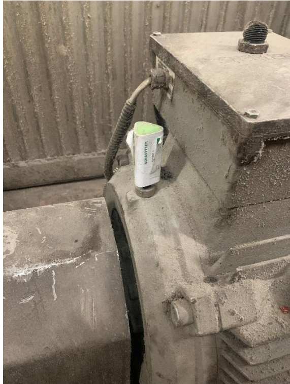
Figure 31: Application of the sensor on the motor's fast shaft output
