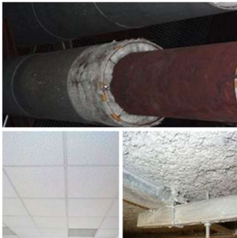
Figure 19: List A materials: false ceilings, tube insulation and flocking
