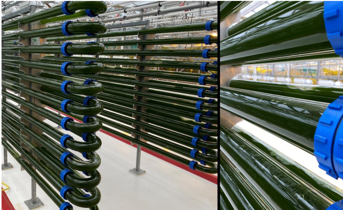
Figure 1.6: Photo of the Lgem photobioreactor discussed in this Thesis in operation.
