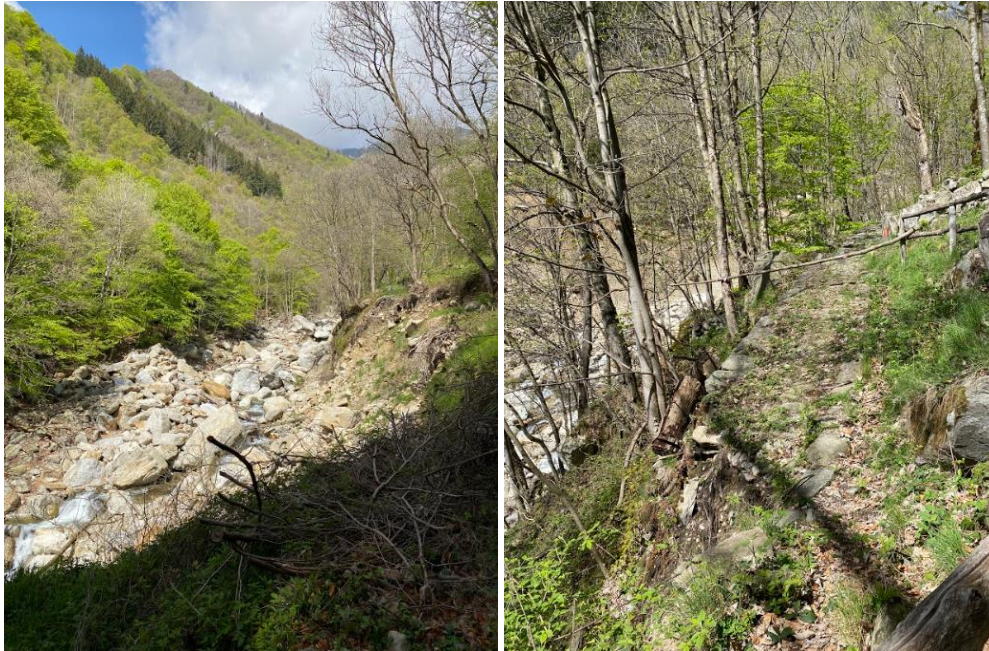
Figure 7. Landslide of River embankment and Closure of Pedestrian walkway due to landslide
