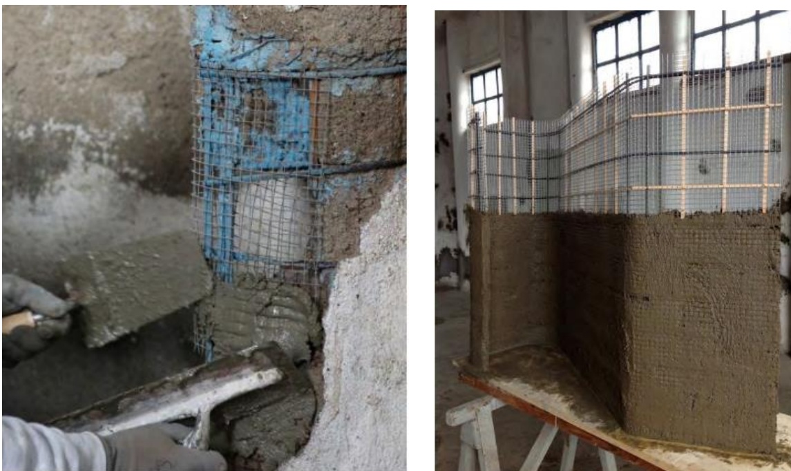
Figure 38 Full size model of a portion of the Magliana Warehouse's curly wall, 2013 (Photo Sergio Poretti, SIXXI Project) (LEFT), Magliana Warehouse. Restoration works, 2013 (Photo Sergio Poretti, SIXXI Project). (RIGHT)
