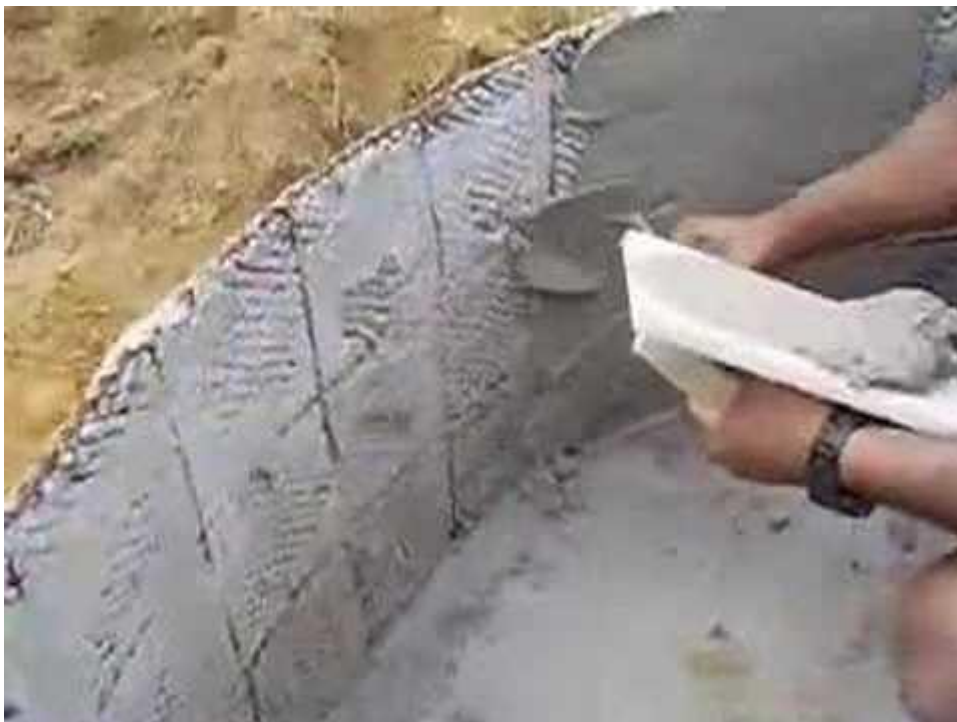
Figure 3 Having been given a cylindrical shape, cement and its components, mortar and steel
