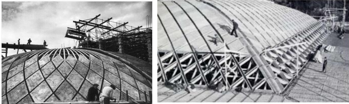
Figure 27 phase of assembling the diamond shape slabs on the vault before casting the ribs [28]
