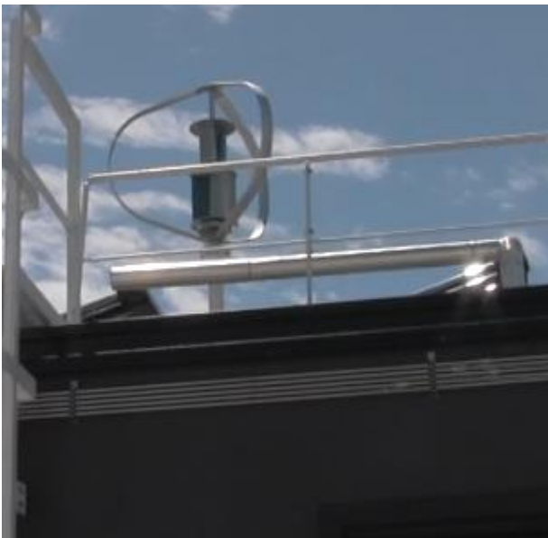
Figure 5-4 vertical axis turbine
