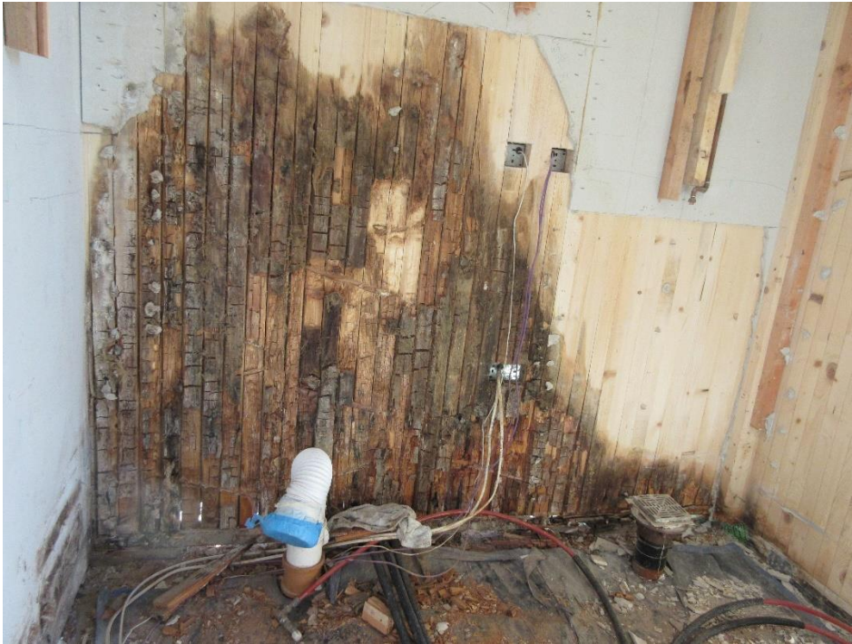
Fig. 58 Water damage on Brettstapel panels
