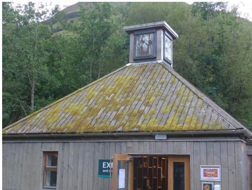
Fig. 20 Wooden roof with moss growth
