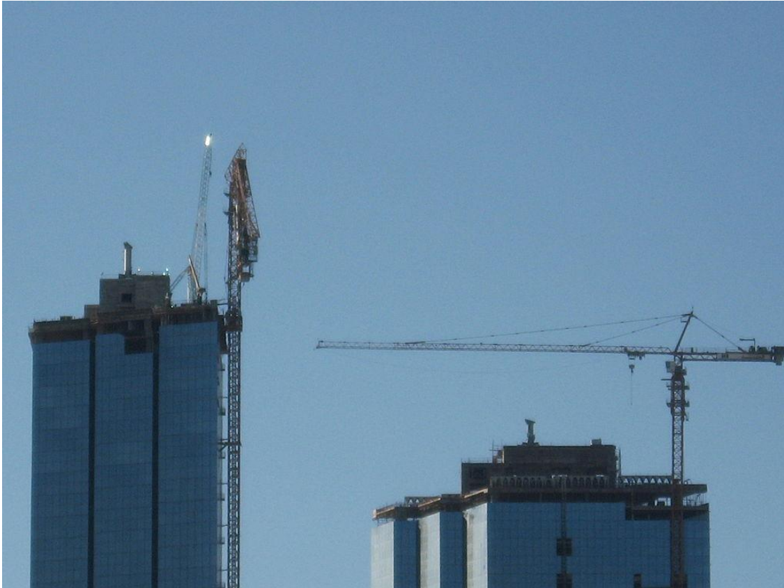
Figure 21: The collapsed construction crane
