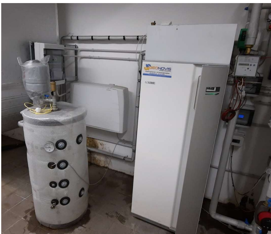
Figure 15: NIBE heat pump of the center with a buffer tank and fan coil
