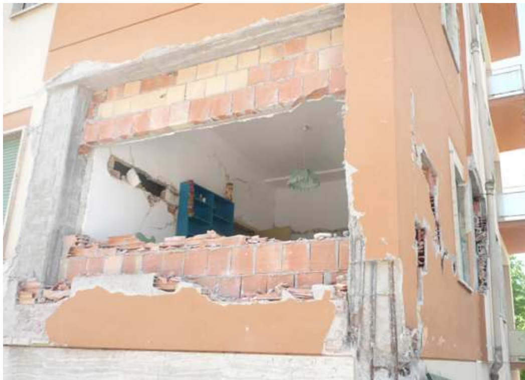
Collapse of the dry wall partition
