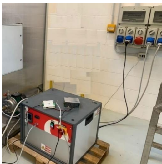
Figure 50 | Furnace power supply.
