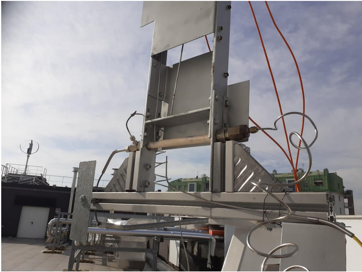
Figure 43 | Alumina reactor on the rooftop of the EC-LAB.
