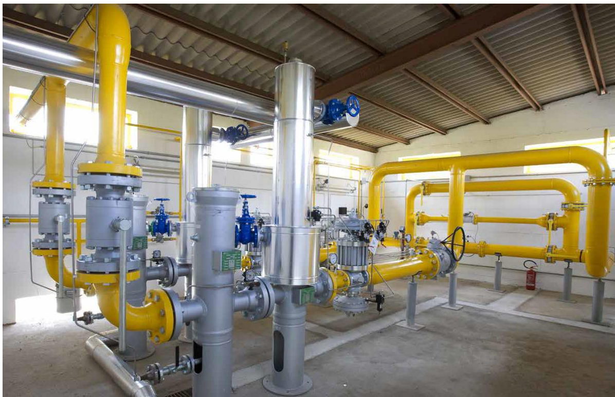
Fig. 1.21 Inside view of a typical pressure reduction station (from [15]).
