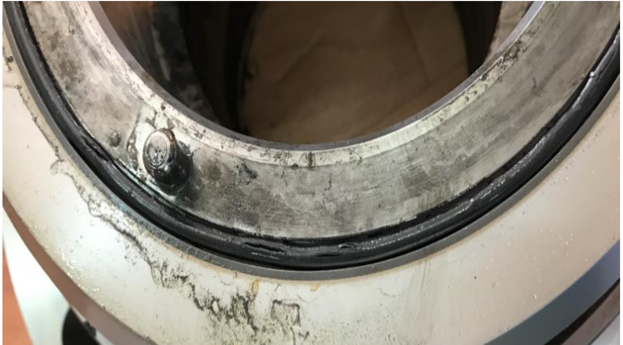
Figure 3.10 Shaft sleeve gasket splitting pattern and tear out
